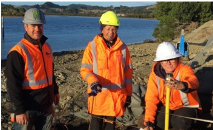
Taipā archaeology from left, lead operator Pip Jecentho and kaitiaki monitor Tina-Lee Yates-Bassett observe project archaeologist Brooke Jamieson investigating and recording a shell midden site prior to removal to make way for new stormwater pipes.
