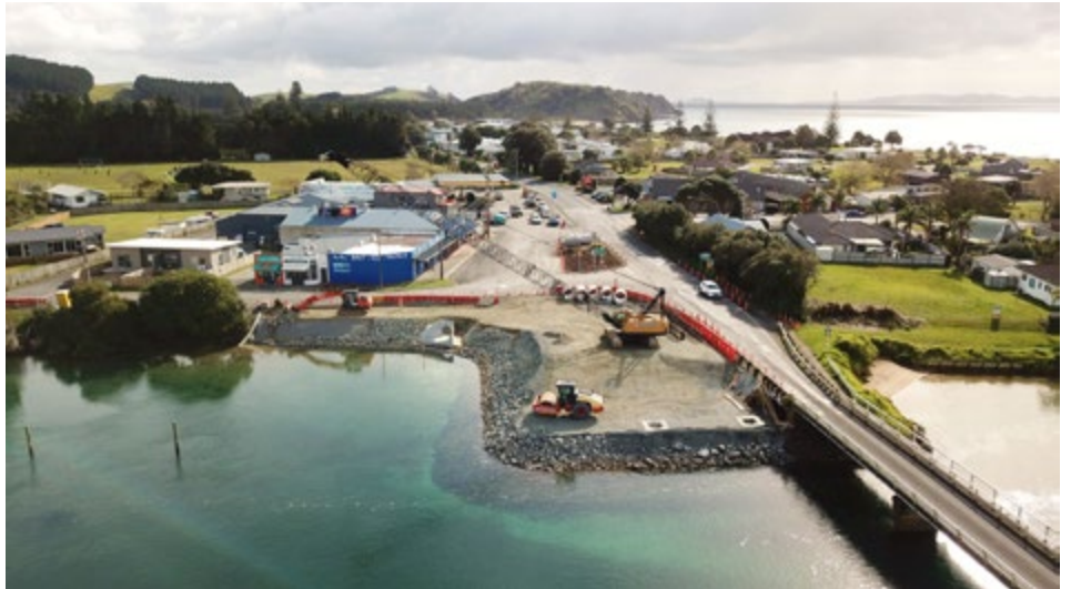
Building the causeway on the township side of Taipā River adjacent to Oruru Road. Along with building the new bridge, a new stormwater pipe is being installed through the shops' carpark and along the side of SH10 as far as Taipā Area School.
