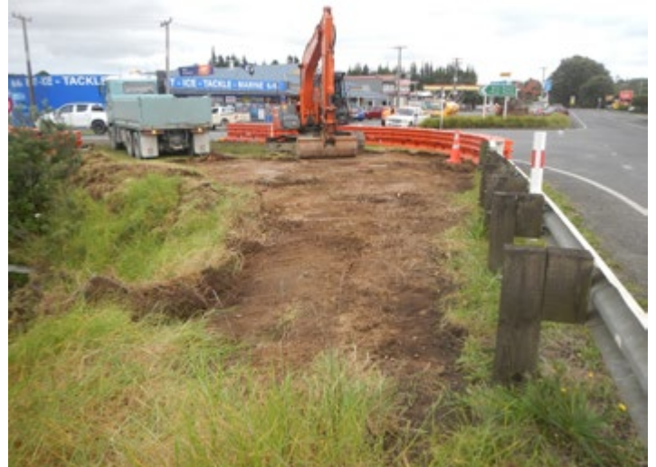
Topsoil stripping: Archaeological monitoring of topsoil stripping on the western side of Taipā Bridge (Source: Clough & Associates Ltd, 2018)
