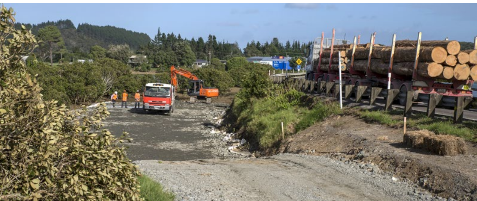
Trucks carrying out excavated tidal mud and bringing in material access site directly off SH10 at the intersection of Taipā Tides Drive. Photo: Malcolm Pullman
