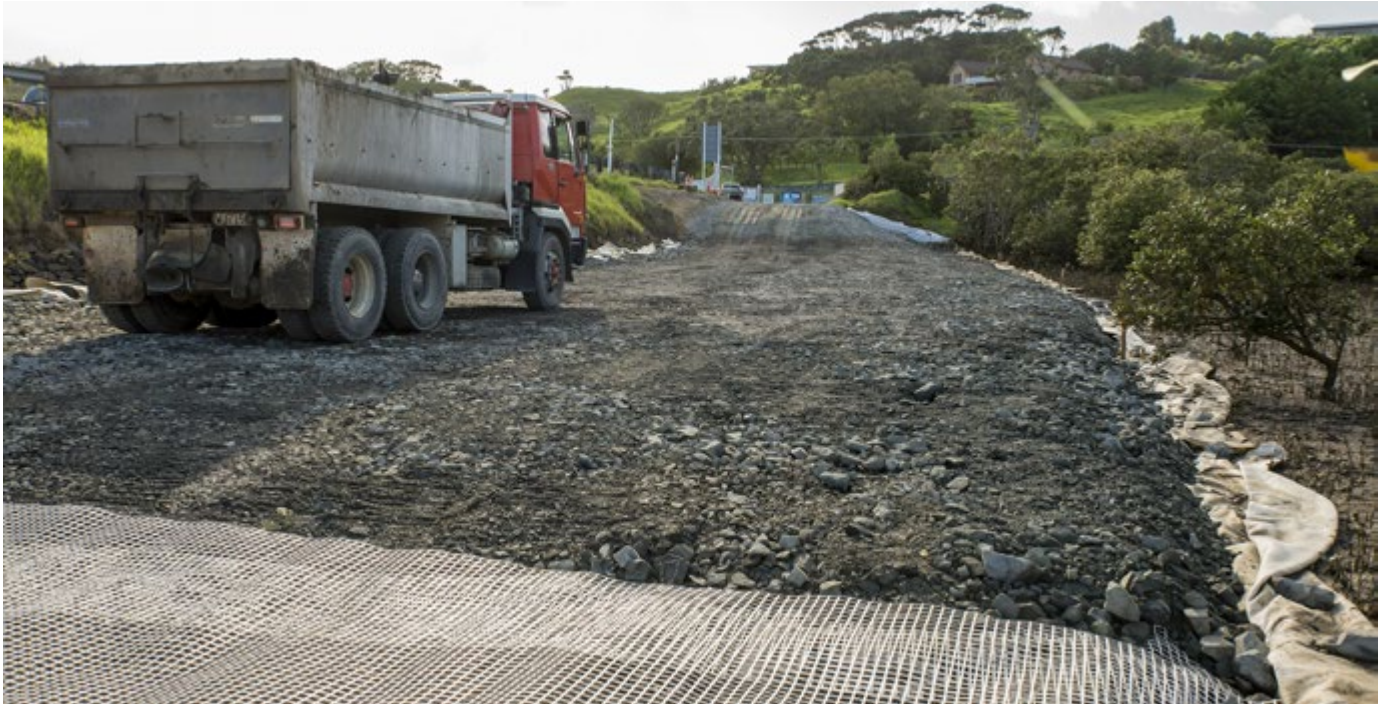
Causeway construction on the east side of Taipā River. Photo: Malcolm Pullman
