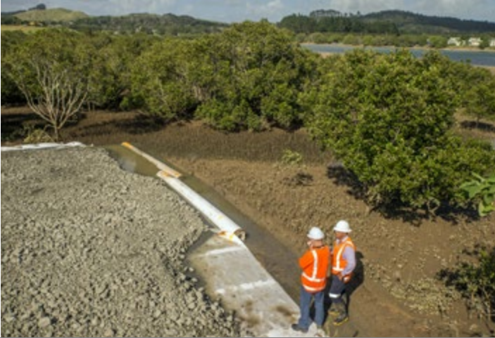
Strong geo-cloth is laid to contain fines (sediment) as layered material is built up to form the causeway. Photo: Malcolm Pullman
