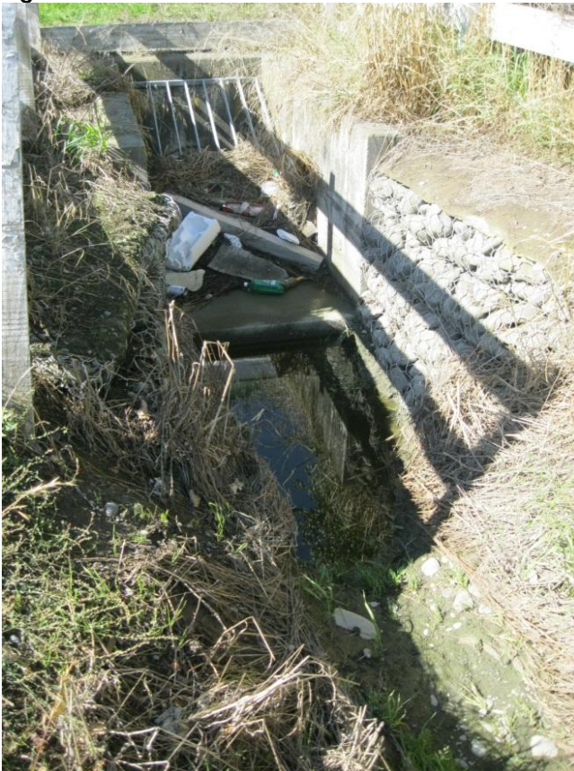
Figure 6 Intake structure on Halswell Junction Road
