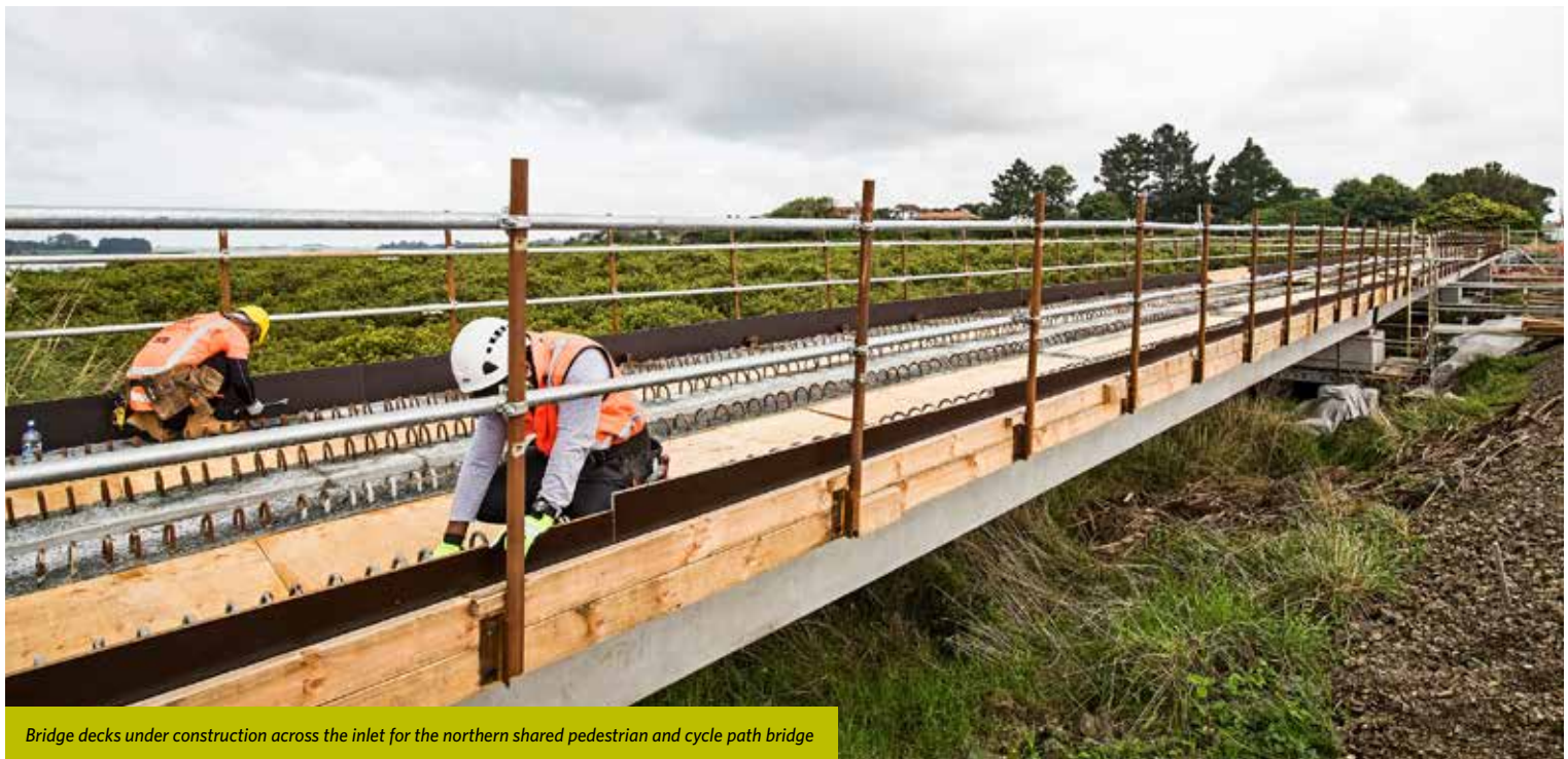
Beams are lowered into place for the shared pedestrian and cycle path bridge
