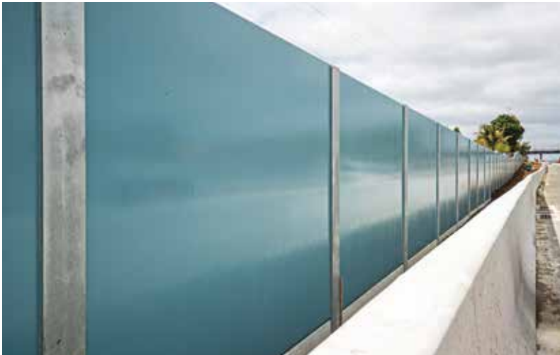
▲ New noise walls in place between Takanini Interchange and the Pahurehure Inlet. All plantings are native and include two types of climbers. Muehlenbeckia – common name Mingimingi and Tecomanthe Speciosa – common name Three Kings Vine.
