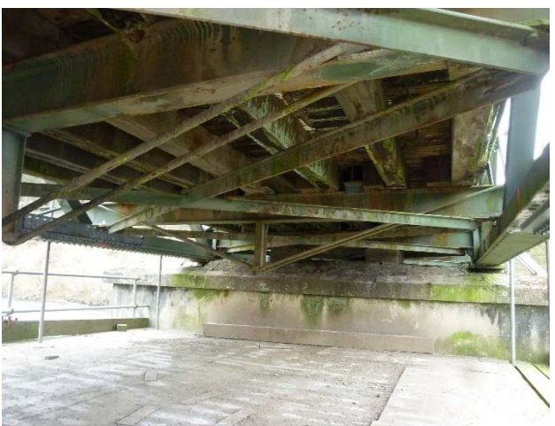
Figure 35: Understructure of the bridge showing king post trusses strengthening transoms and cross bracing below timber deck. Microbiological growth and accumulation of dirt is evident.
