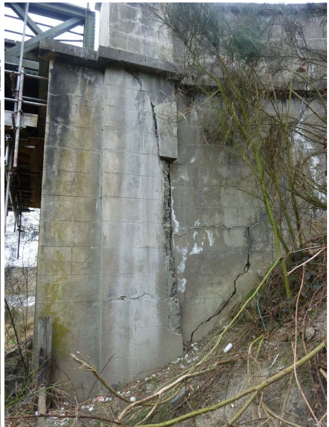
Figure 30: North elevation of west abutment. Serious cracking and delamination of the concrete are visible.
