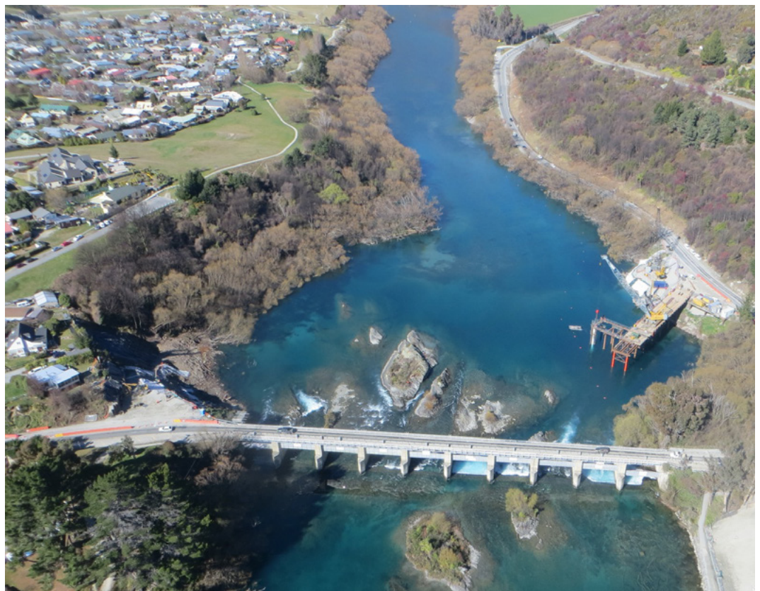
An aerial view of the construction platform needed to build the new bridge edges further out into the Kawarau River.
