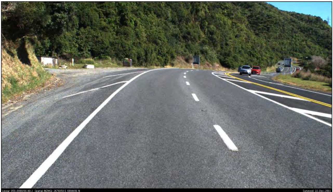
Figure 3-3: Approach to the tight, uphill, right hand curve on Site 2 from the east (Increasing RP 0/1.42)
