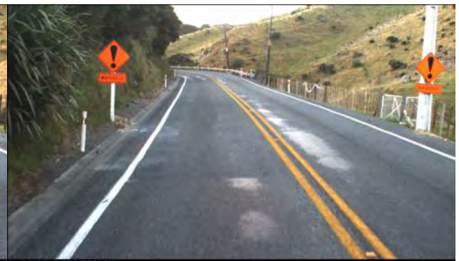
Figure 3-6: Approach to 'Washout' area and second curve in the 'broken back' alignment heading west (Increasing)
