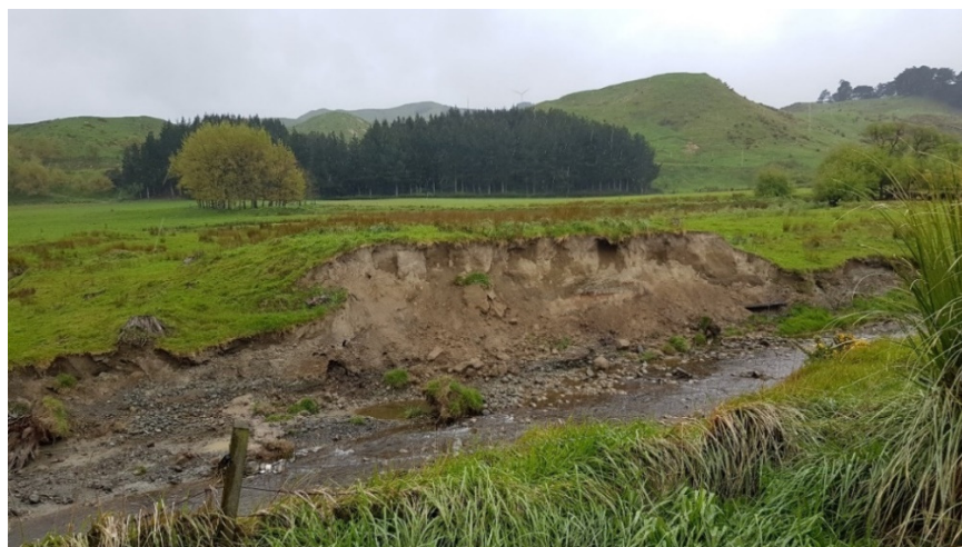
Figure D.55: Mangamanaia Stream showing typical bank collapse and the material comprising the bed and banks.
