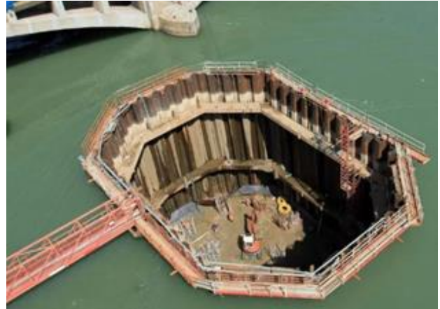
Figure 16 Te Ahu a Turanga Technical update workshop 221119 - River bed access via coffer dam structure
