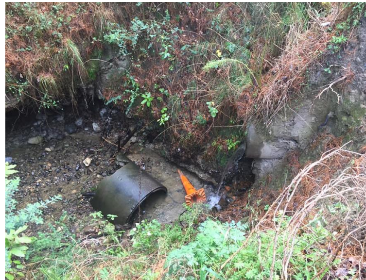
Figure 26 Site visit - broken culvert spotted
