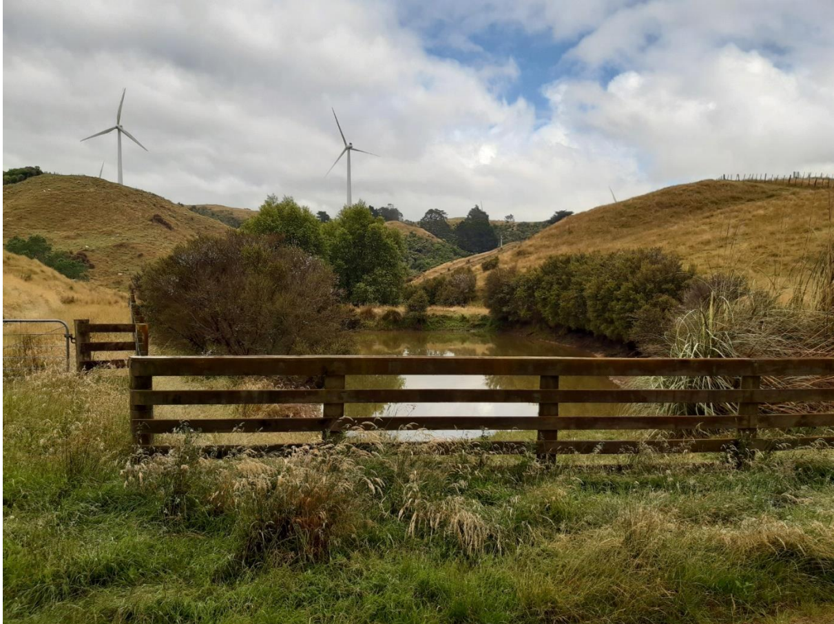
Spoil Site 1 looking towards the top of the range towards the Meridian complex
