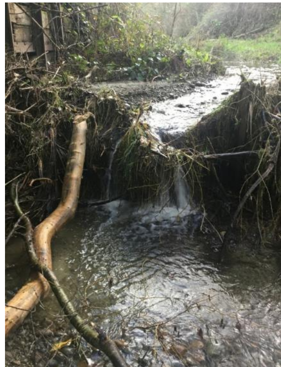
Image 6.C.34: Downstream reach of the main stem (7A). Note the stream flowing over a retaining wall structure reducing fish passage.
