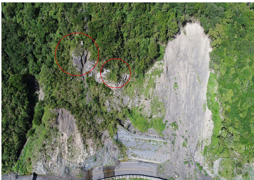
Figure 3 – Photograph of Kerry’s Wall Slip from western side in February 2018 (Source: NZ Transport Agency website) - the red circles indicate cracks above Kerry’s wall, which are areas assessed as being highly vulnerable to future slips
