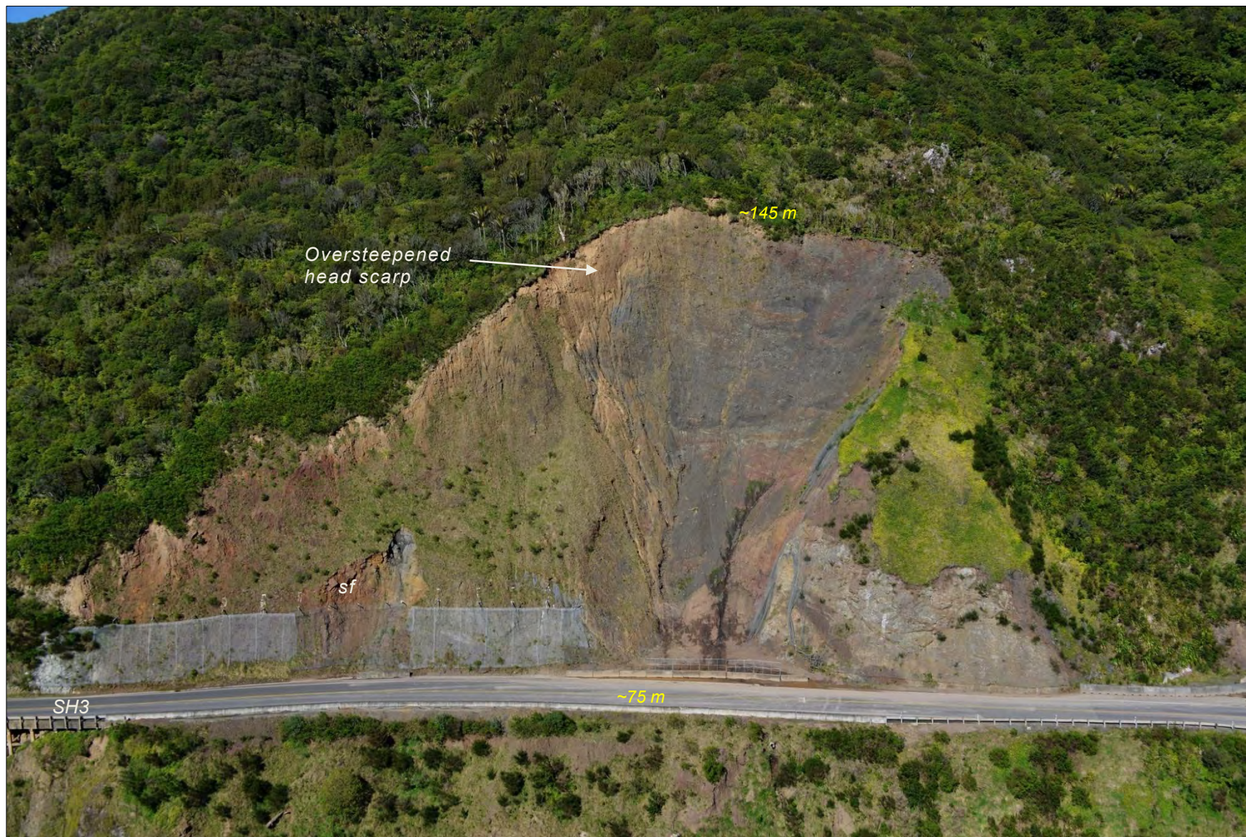
Figure 17. Closer view of the 2004 landslide #2, the largest potential landslide site (Area 14). A small failure ( sf ) on the lower slip face in July/August 2012 removed part of the rock fall mesh. Bedrock at this site is weak, closely jointed, weathered red argillite overlain by thick colluvial deposits. The steep ( 45\text{--}60^\circ ) head scarp now extends \sim 70 m above SH3 and is likely to retreat further upslope in the future. Open tension cracks are present \sim 20 m above the head scarp.
