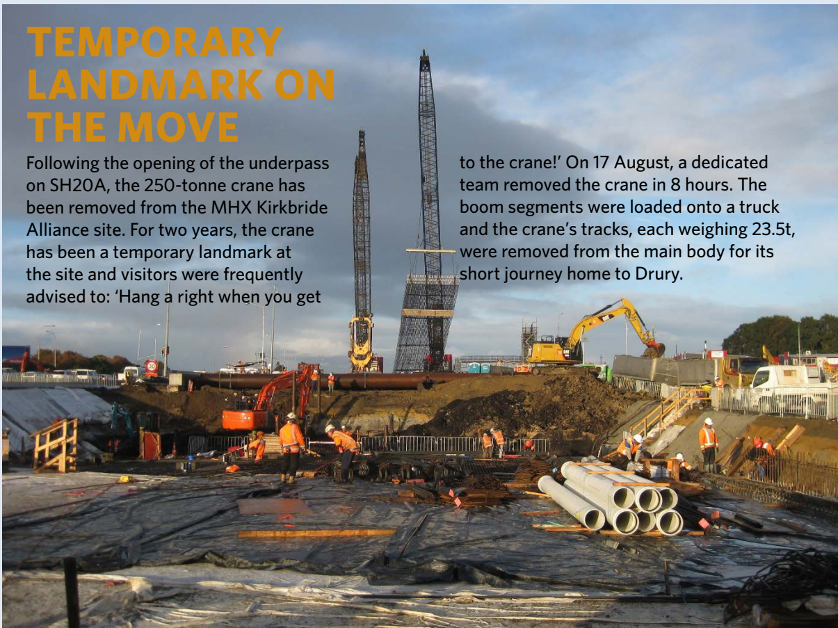
The 250 tonne crane shown to the right lifts reinforcing into place in the underpass.
