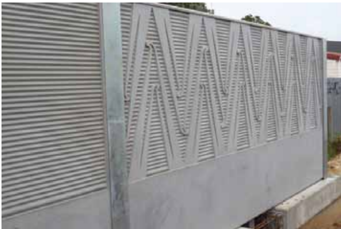
Noise walls northbound on-ramp will be complete by the end of March; you can read more about the noise walls over the page.
