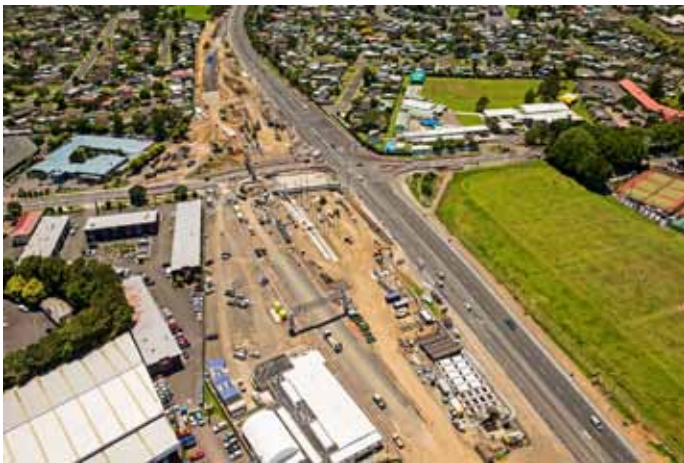
The project looking north along SH20A. A picture is forming of where the northbound ramps and trench will be.
