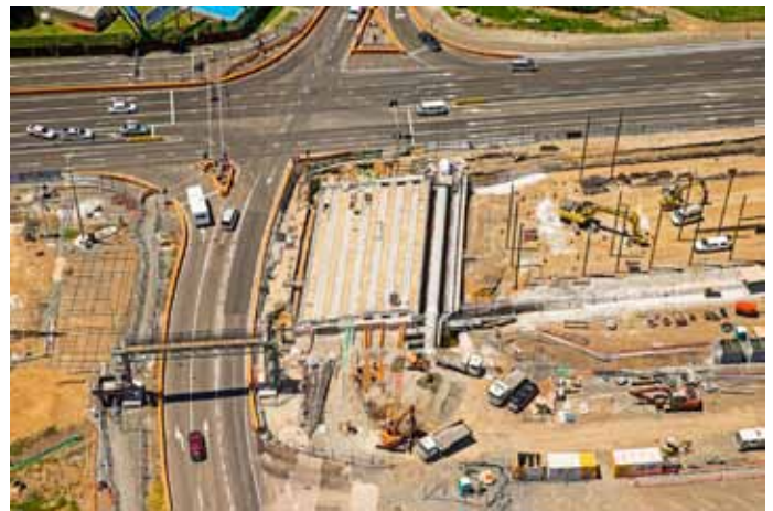
The southern half of the Kirkbride Road bridge. The Hunua 4 watermain can be seen running along the far right edge of the bridge.
