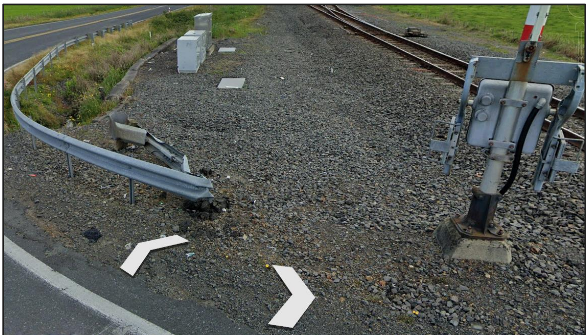
Figure 4-9: Damaged terminal on Northbound approach
