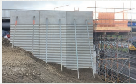
Pre-cast panels with piles behind in place to support the new Royal Road Bridge structure.
