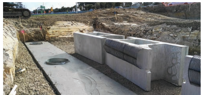
Piles will be augured (drilled) into the circular holes and concrete infilled, once the stone strong blocks (on the right) are in place. Photo taken next to the Royal Road off-ramp. A noise wall will be constructed on top.
