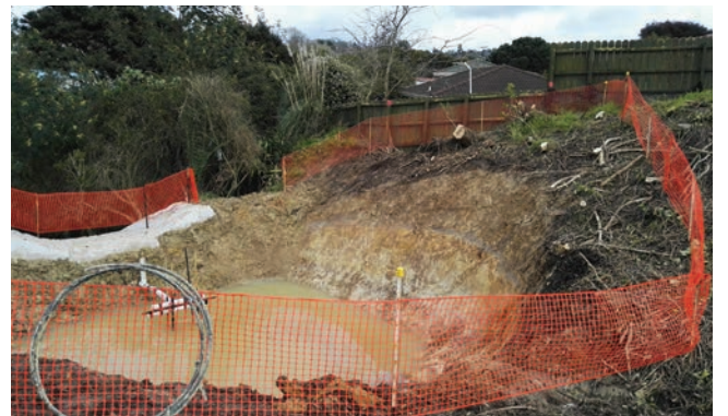
One of the three temporary decant treatment ponds that are on site.
