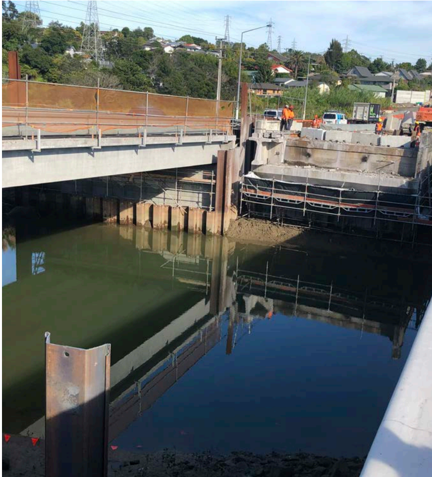
The gap where the old bridge used to be with traffic now running on the first half of the new bridge.
