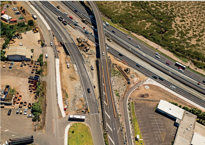
In December 2015 the Patiki Road on-ramp and two lanes westbound were moved. Work continues on the cycleway underpass.
