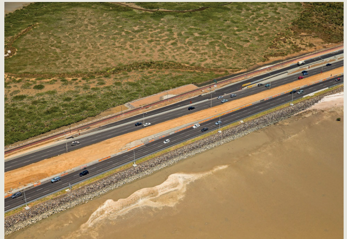
In January the team moved the Rosebank Road off-ramp and the express lane westbound. This photo shows the new off-ramp area just before it opened to traffic.
