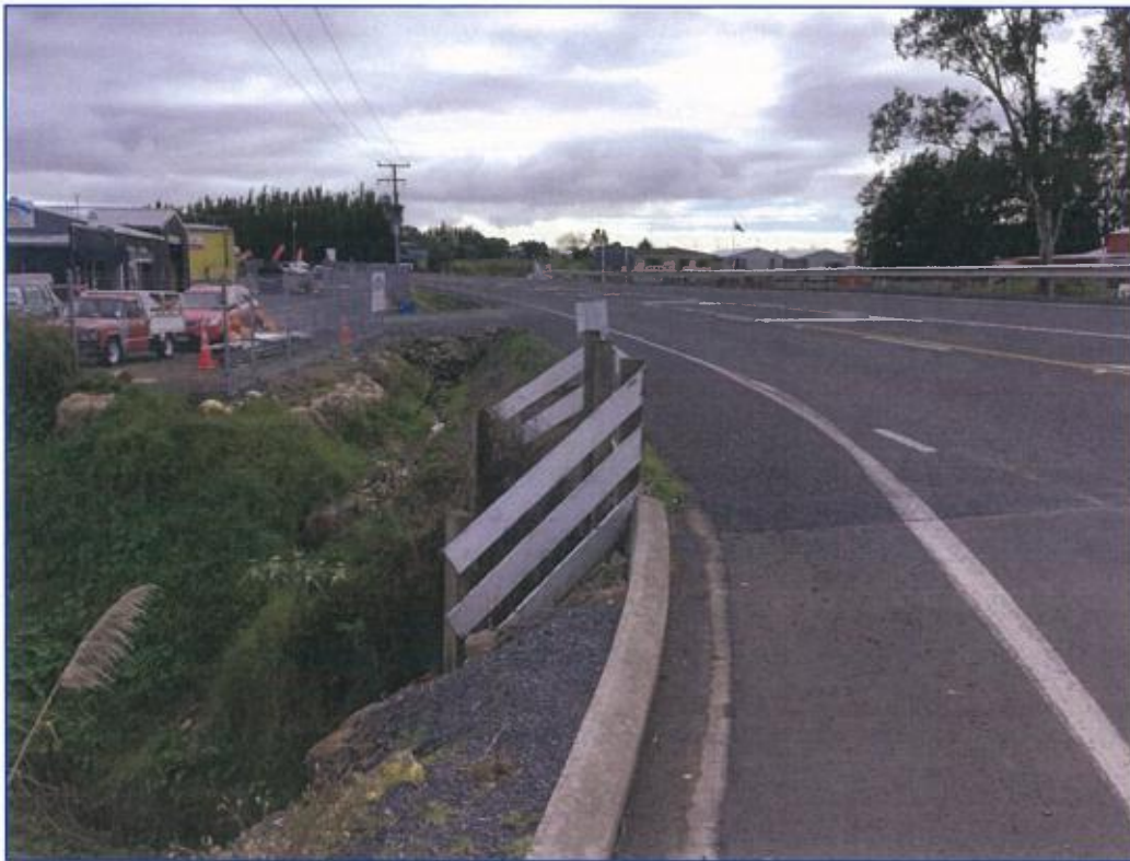
Figure 14: The Whiriwhiritoa Stream Culvert No.730 that is unprotected on the upstream (western) side.
