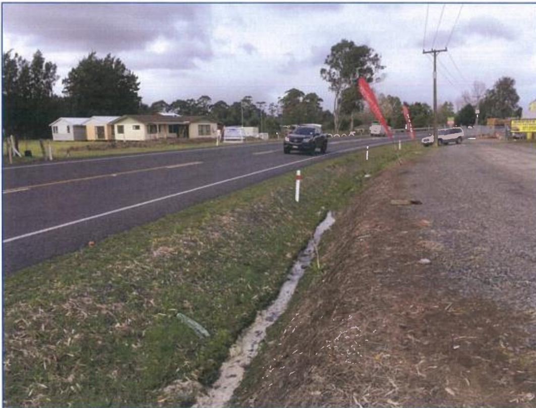
Figure 13: The open drains along the western side of SH10, south of Skippers Lane.
