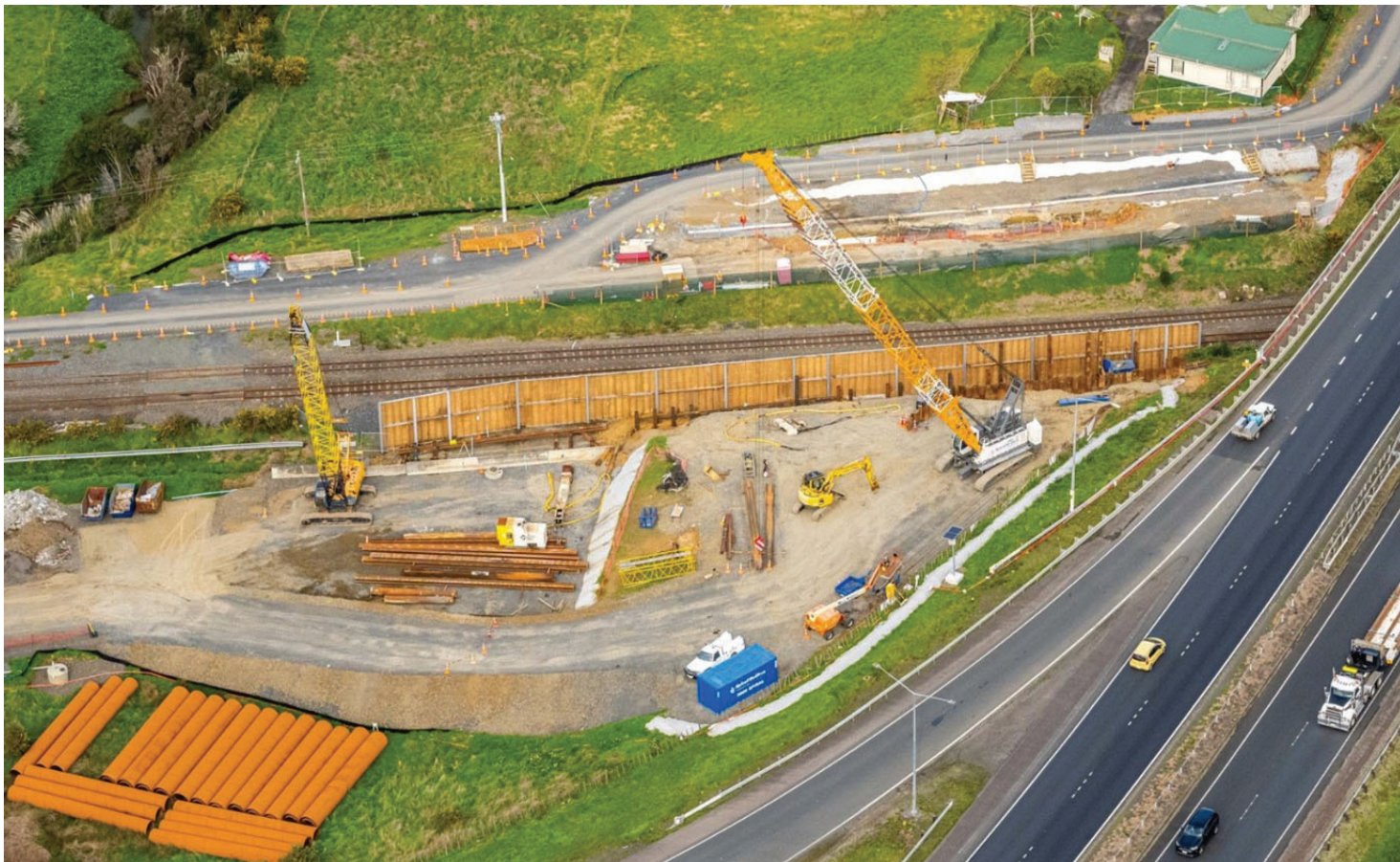
Replacement motorway bridges across the railway are being built from Karaka Reserve within Drury Interchange across to Flanagan Road. In the image above, piles are being driven in behind a large hoarding fence on one side of the railway lines. In the image below, a reinforced concrete 'upside down U' is being built to protect an arterial watermain on the Flanagan Road side.
