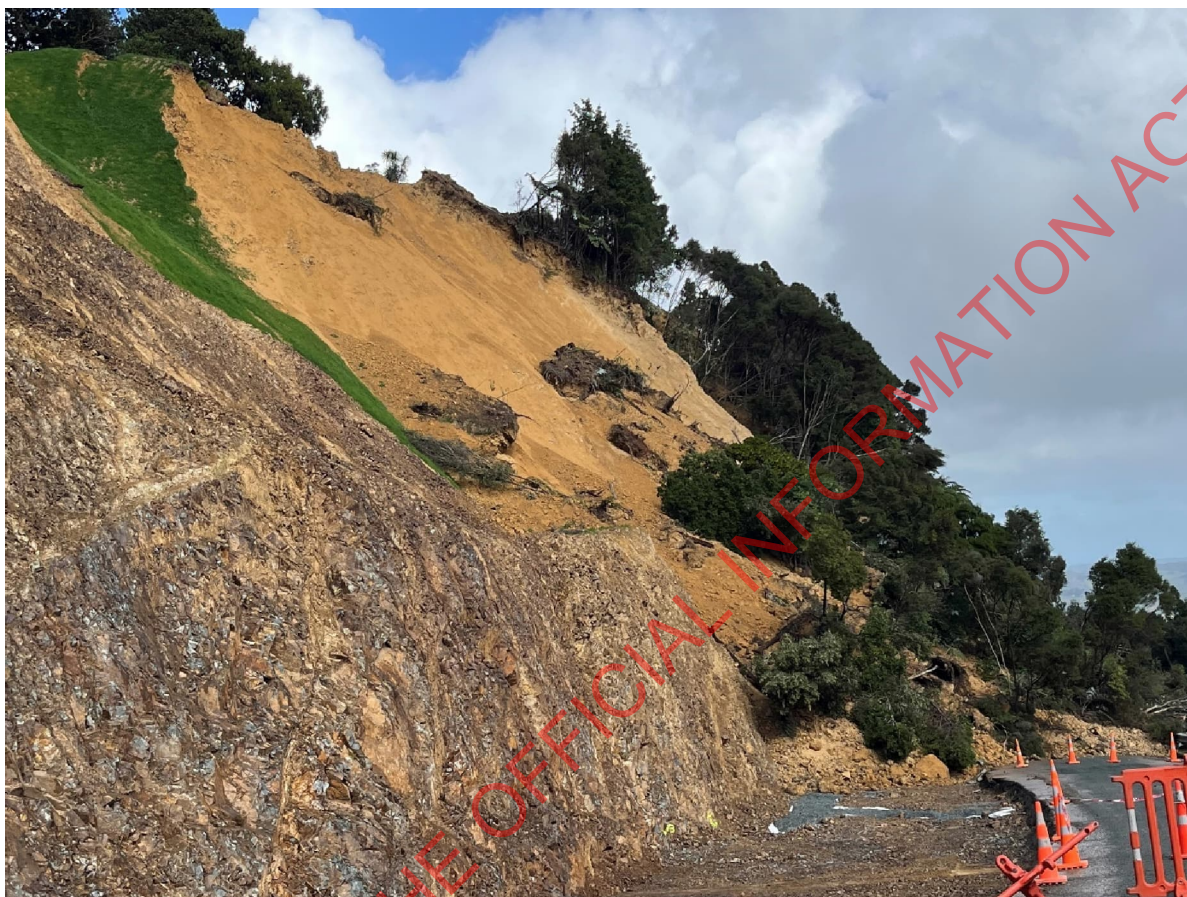
Figure 4: Landslip showing debris at road level and evacuated face above. HW rock exposed in foreground and hydroseeded face of earlier failure in Section D above with cracking evident at crest. HW rock is present at mid-height of the evacuated scarp.
