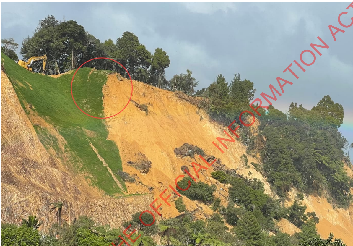
Figure 3: Failure scarp showing over-steepened rear scarp at crest and cracking circled behind the crest where it is exposed in the adjacent side face of the earlier landslide in Section E.
