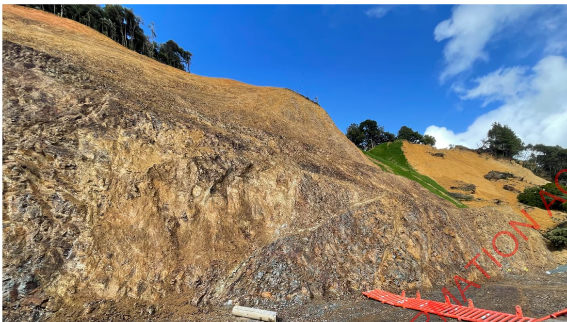
Figure 2: Section F in foreground and Section F beyond showing the recent failure in this section. Sections are on the west facing slope on north trending spur ridge with a series of steeply incised gully features (see Figure above, the recent slip is on the right of the photo).
