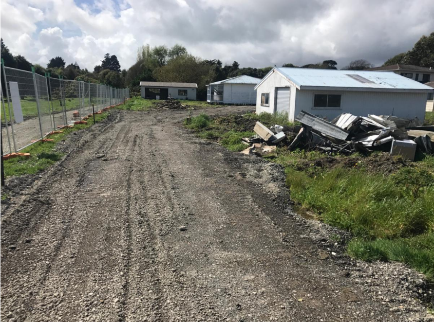
Driveway running along the western boundary of the site, taken from the western corner, facing north east (photo taken: September 2017)
