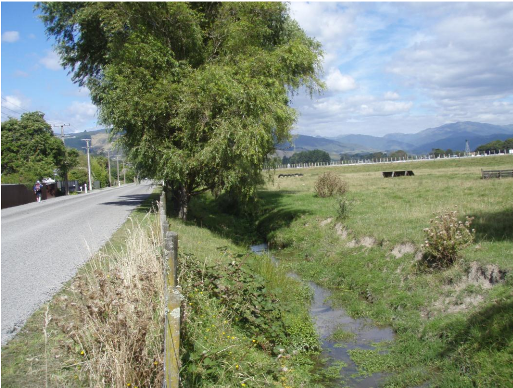
Figure 2-1 Drain along north side of Ōtaki Racecourse directing storm runoff into Mangapouri Stream (viewed looking east from site of culvert under Rahui Road to Mangapouri Stream)
