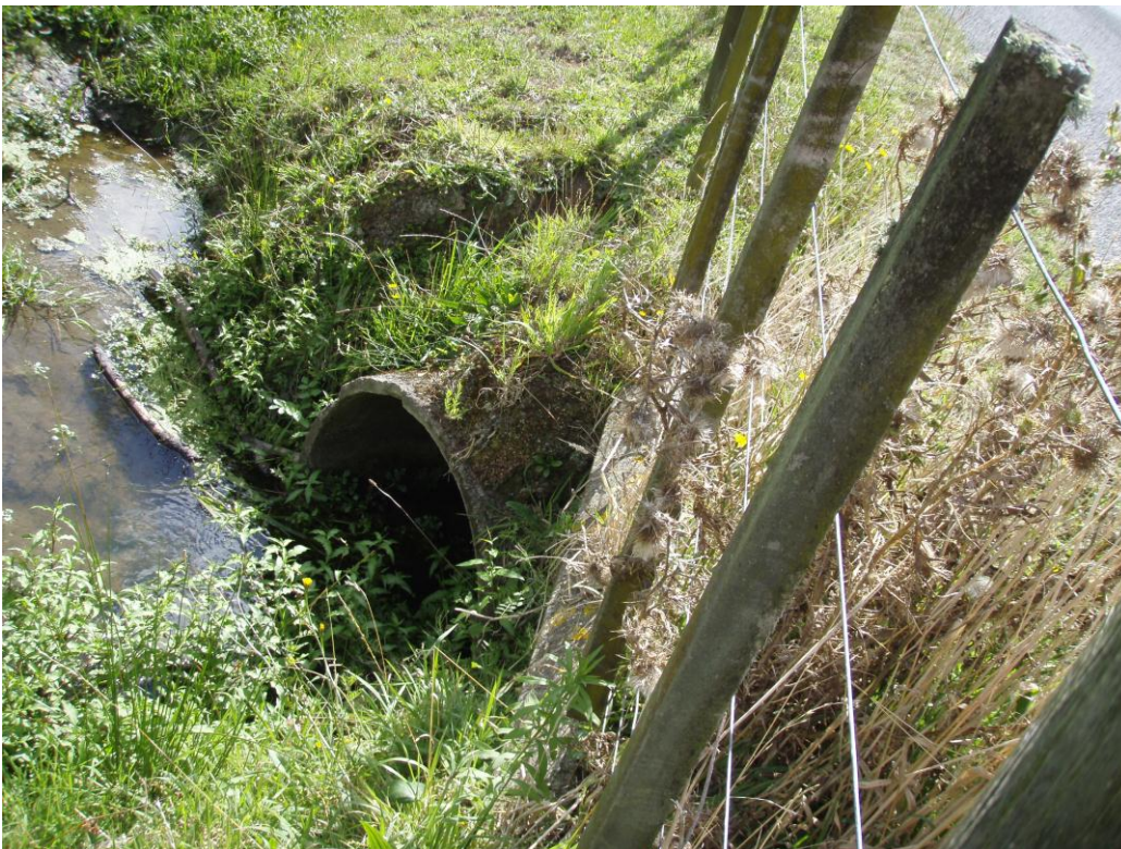
Figure 2-2 Culvert under Rahui Road directing storm runoff from Ōtaki Racecourse to Mangapouri Stream
