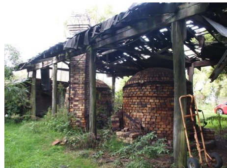
Figure 24 kilns and flue with clay preparation shed to the left, photo I Bowman, 11 May, 2012
