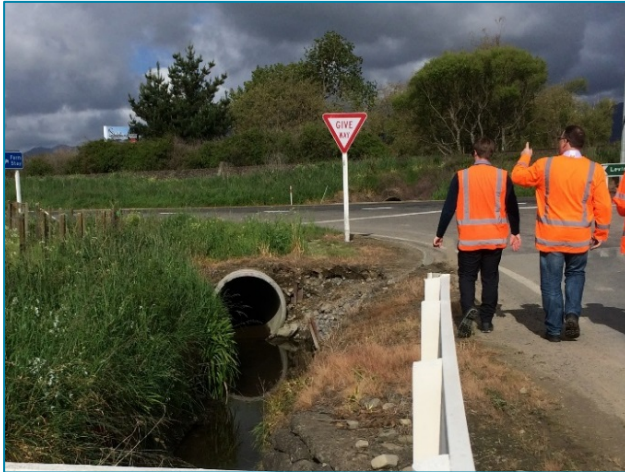
Figure 2-21: Buller Rd Culvert (hazards on both sides of SH1 and Buller Road)
