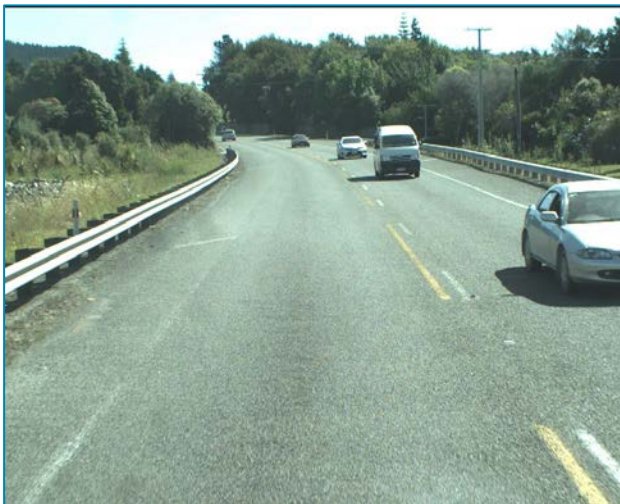
Figure 2-10: Faded line marking
