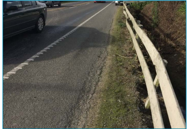
Figure 2-18: Deep drain and failing retaining wall south of St Stephens Church
