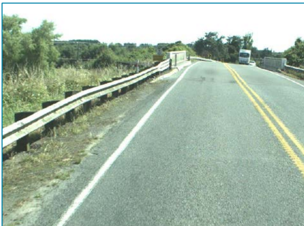
Figure 2-15: Narrow sealed shoulder and non-compliant bridge barrier, Ohau Rail Overbridge
