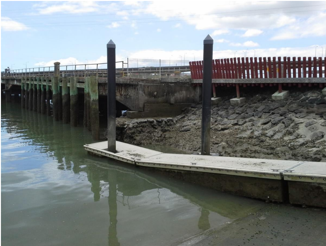
Figure 36: the southern abutment looking north from the boat ramp. Photo Matthew Felgate.
