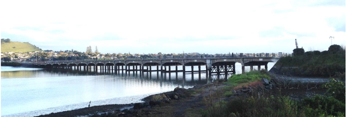
Figure 22: View of the Old Māngere Bridge Looking towards Māngere. Matthews & Matthews Architects Ltd 2014.
