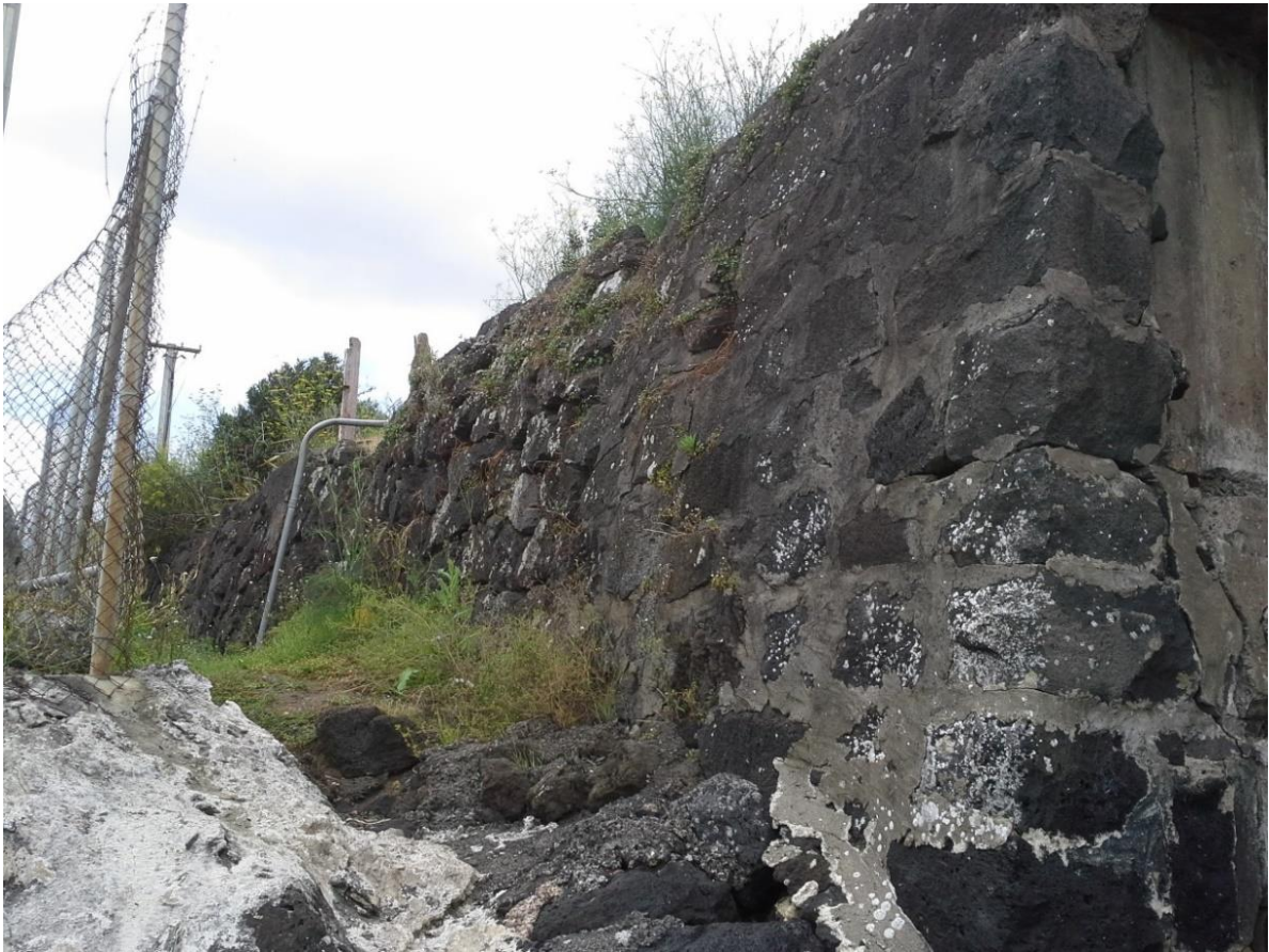
Figure 40: The western side of the northern embankment has a more vertical basalt/scoria retaining wall. Photo Matthew Felgate.
