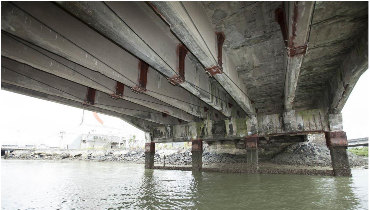
Figure 32: View towards north end showing significant deterioration to side beams. Fraser Newman Photography.
