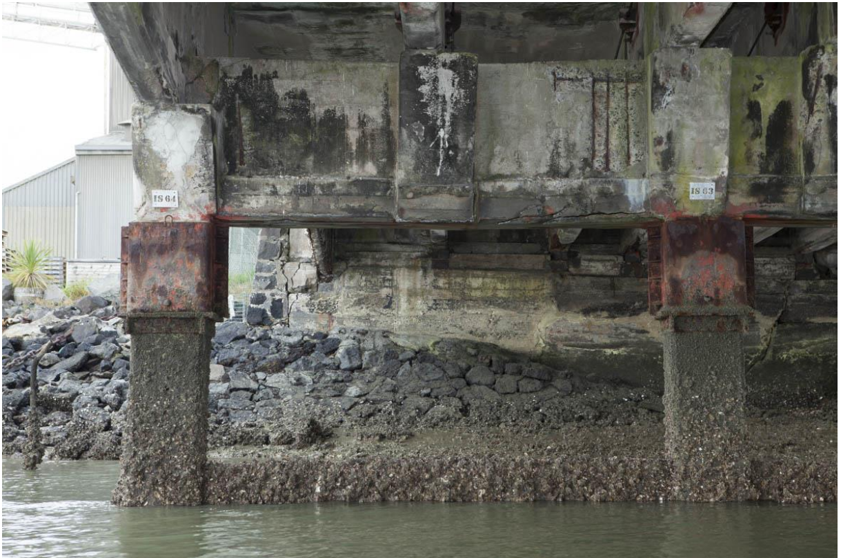
Figure 31: View to north end, showing significant deterioration and various repairs. Fraser Newman Photography.
