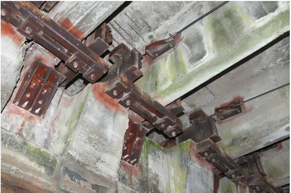
Figure 34: View of some of the repairs undertaken to the underside of the bridge. Fraser Newman Photography.
