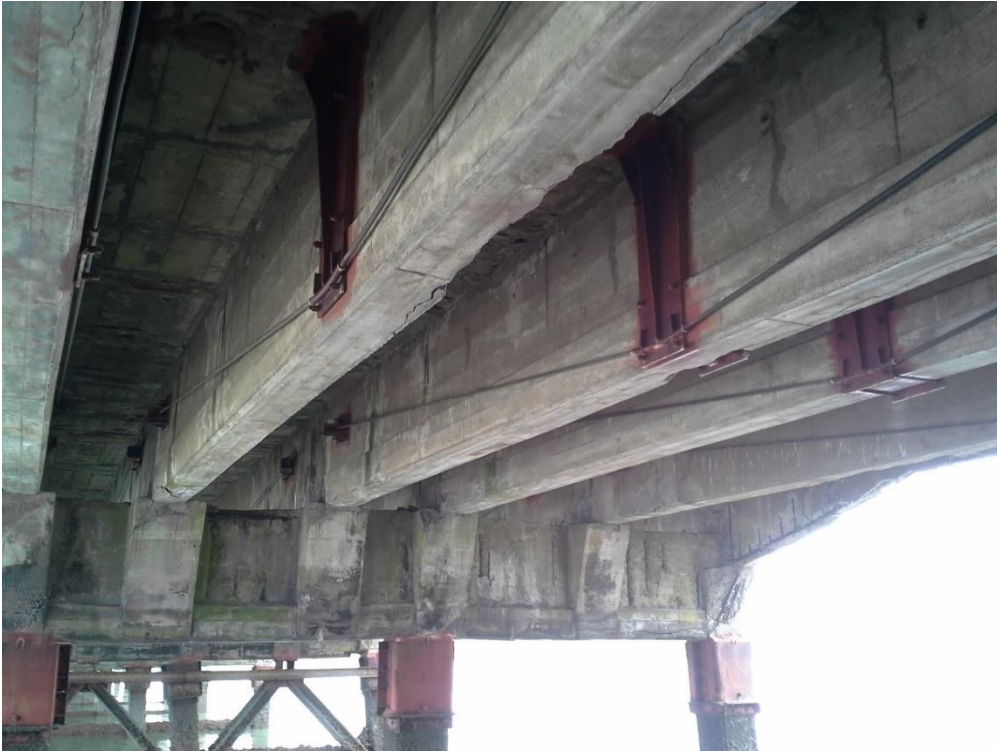
Figure 28: View to underside of the bridge showing the parallel girders spanning between the main beams. Strengthening to the girders is visible. Dr Matthew Felgate 2017.
