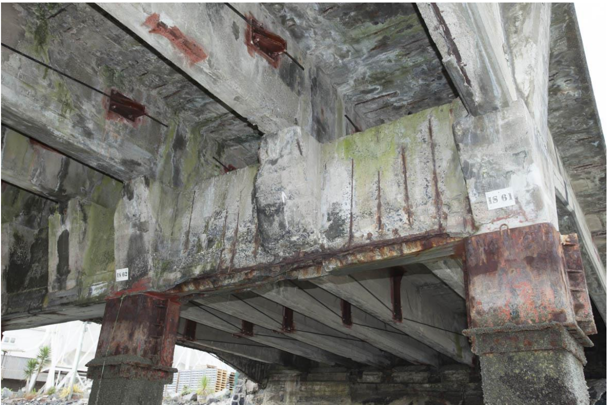
Figure 30: Repairs to column caps and beams and deterioration to beams and underside of deck. Fraser Newman Photography.
