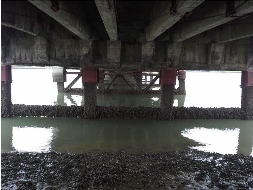
Figure 26: View to underside of the bridge showing the parallel girders spanning between the main beams, supported on four piles. Cross bracing added to strengthen the piles is visible. Dr Matthew Felgate 2017.
