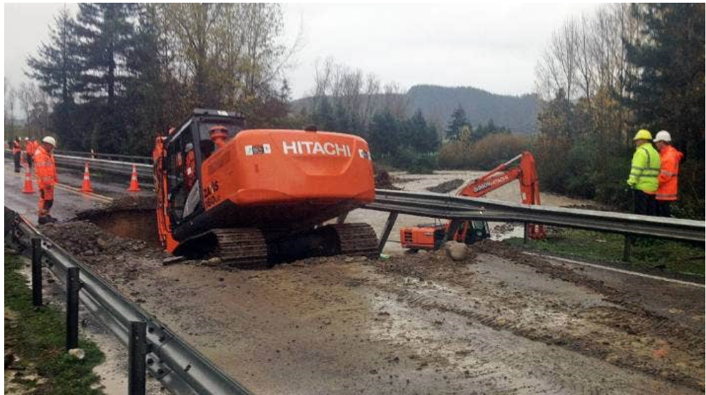
Figure F.8: Damage to Waikawa SH1 bridge left bank June 2015 upstream view (photo Joel Maxwell, Stuff.co.nz)
