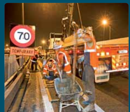
SLOW DOWN OVER NEWMARKET. To enhance safety while keeping Auckland moving, new speed limits and barriers are now in place across the Newmarket Viaduct.
