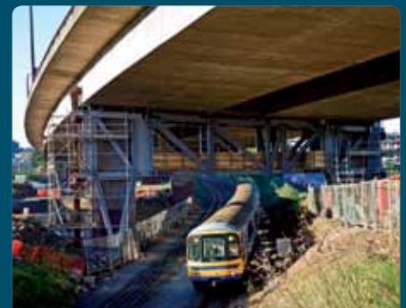
KEEPING AUCKLAND MOVING The steel supports were installed at Easter, when the rail line was closed, to avoid causing further disruption to Auckland's transport network.
