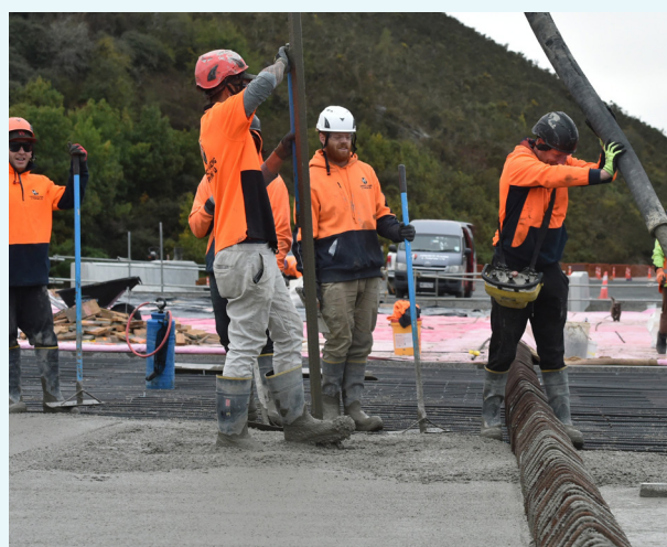
Crew busy with the final concrete deck pour completed in April. Photo supplied by the ODT
