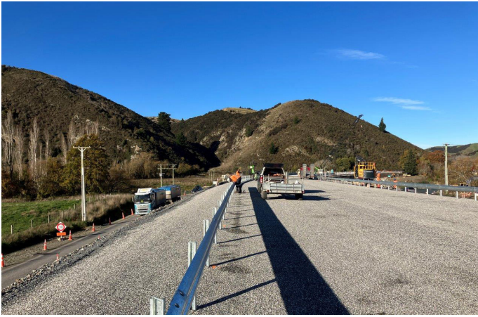
Safety barriers being fitted on the western road approach to the new bridge
