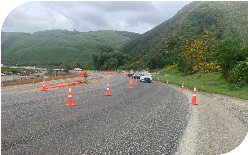
Taking a new approach – traffic travelling on the eastern road link to the new bridge
