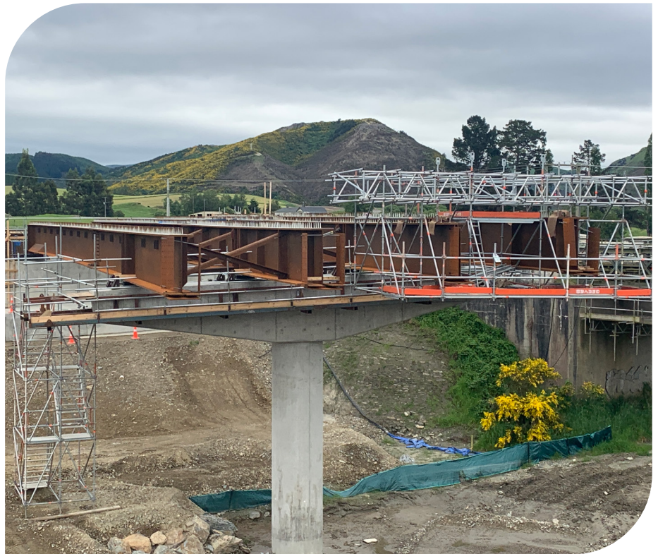
Scaffolding on the western side of the bridge to enable construction crews to splice (bolt) structural steel beams
