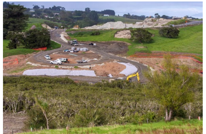
Taken from the east end of the new road alignment, looking westwards to where a haul road has been installed to provide access to the tidal estuary that Bridge no.2 will span, with the limestone quarry in the background.
