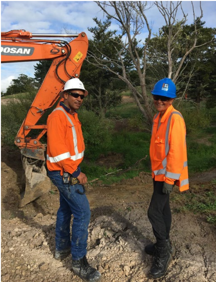
Site Foreman Tia Walters (left) discusses excavation works with Kaitiaki Monitor Ngahua Wright.
