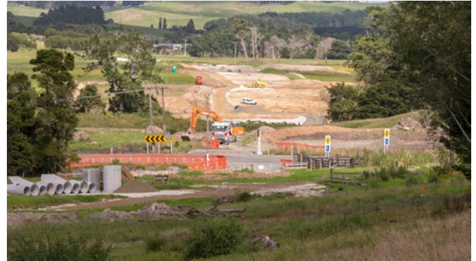
Looking across to the west end of site where a haul road has been installed to provide access to the tidal estuary that Bridge no.1 will span.
