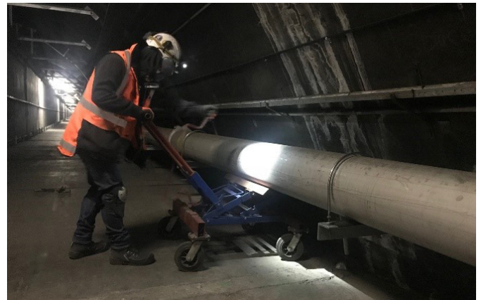
Moving the last section of the new Lyttelton water main into position.
