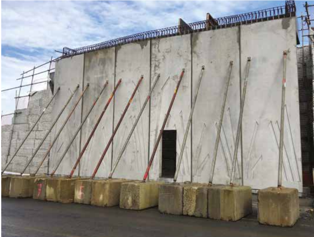
The western abutment wall on the overbridge has a pattern designed by local iwi.
