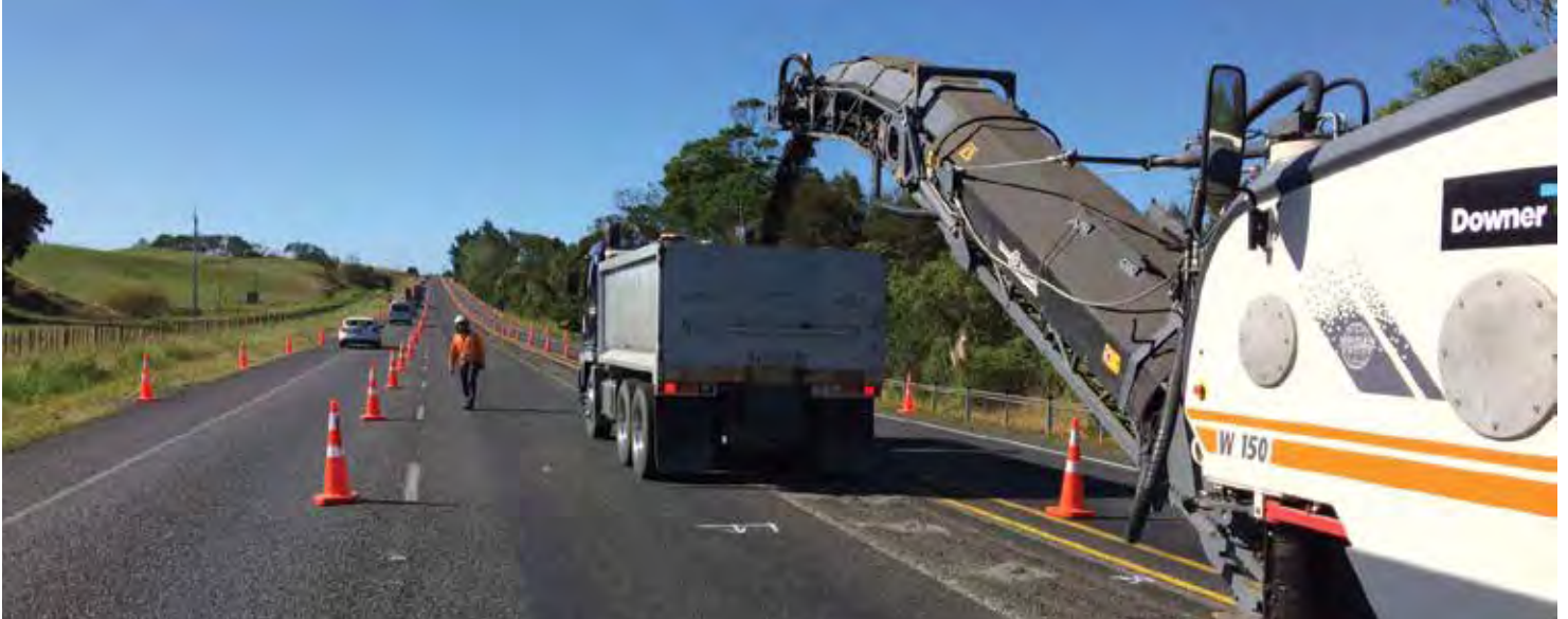
The median barrier is being removed as construction work gets under way
