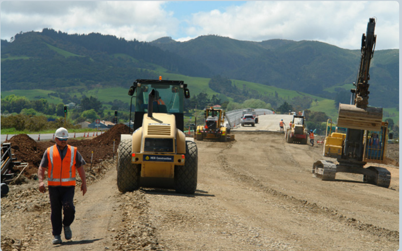
The western approach road is taking shape quickly. Settlement targets have been reached in the critical abutment areas where the approach roads meet the bridge. Road formation and sealing is progressing well due to the warm, dry weather.
