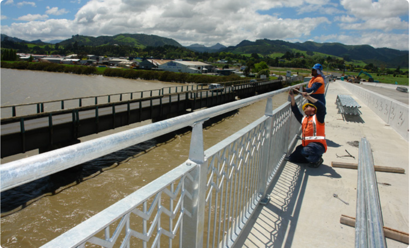
Finishing works on the new Kopu Bridge are progressing rapidly. Here, hand railing on the northern side is near completion.
