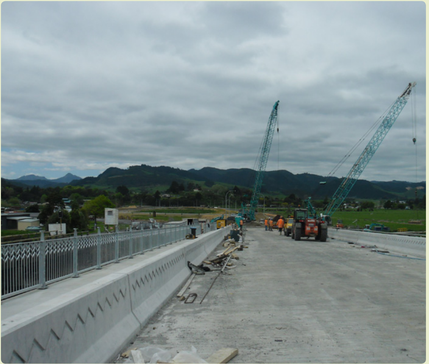
Concrete barrier construction is now complete on the bridge. In the background, the last pair of big cranes complete their final work in late October before being transported off the site. Metal guardrails are still to be fitted on the barrier on the left.
