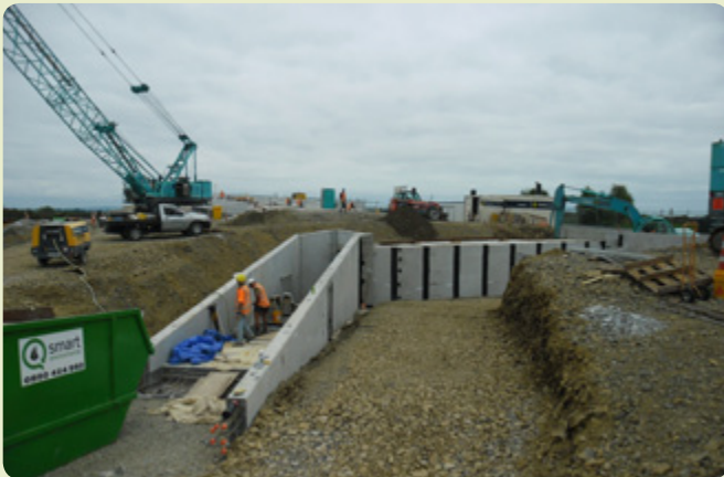
A cycle and pedestrian underpass has been constructed near the eastern end of the new Kopu Bridge. This will provide safe access for cyclists riding the Hauraki Rail Trail cycleway soon to be constructed between Thames and Paeroa. It also links the Rail Trail with the cycle-walkway crossing the bridge.
