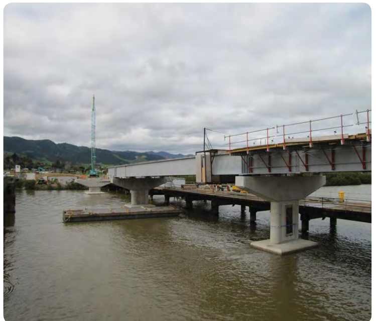
All the concrete piers that support the bridge are finished and the final bridge beams are about to be laid
