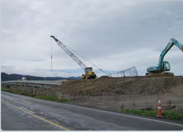
Concrete trucks and construction vehicles can now drive on to the bridge from the western end
