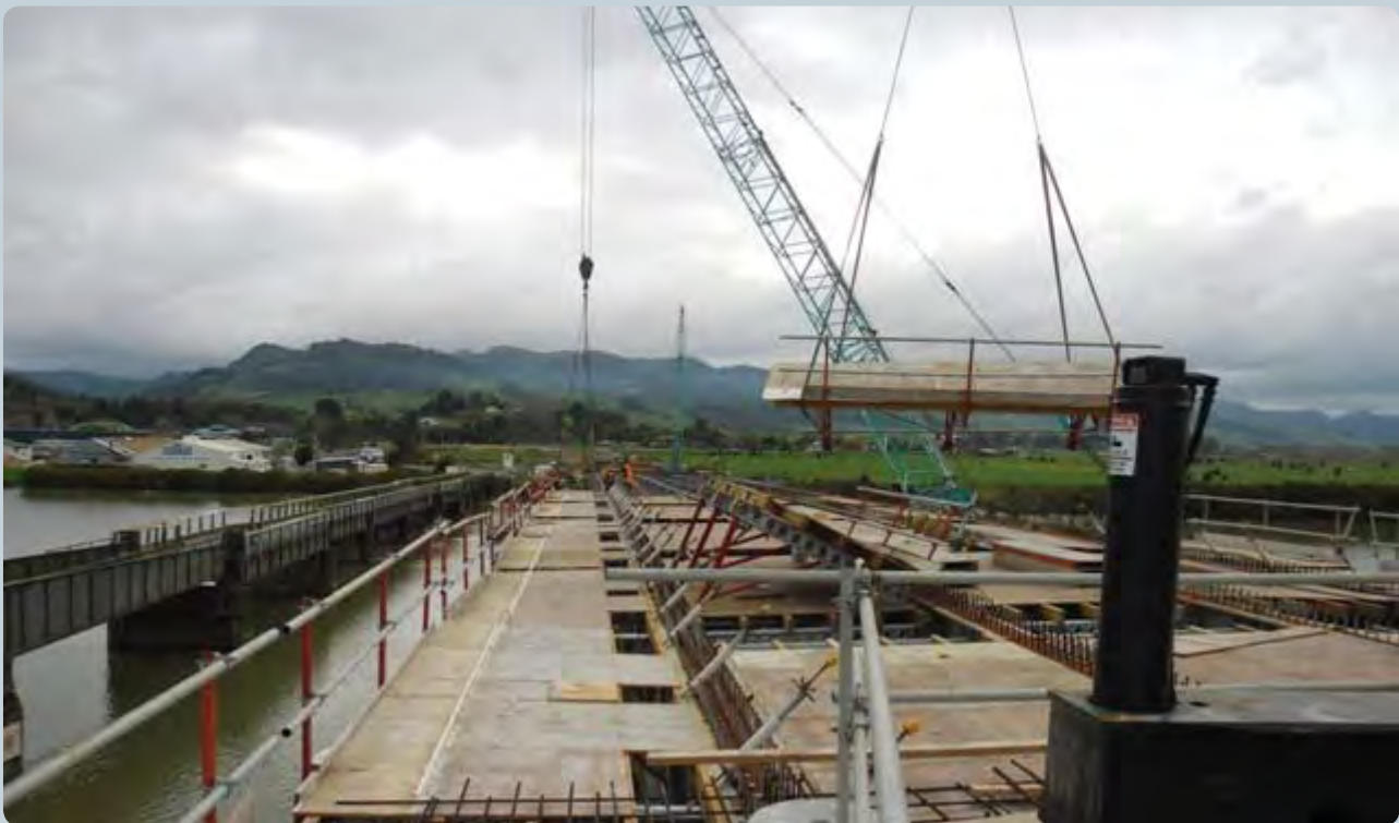
Wooden formwork is placed on top of the bridge beams to form the mould for a new section of bridge deck
