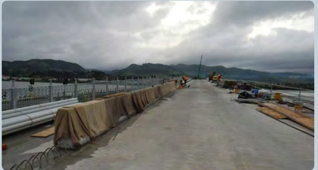
The barrier separating traffic from cyclists and pedestrians is under construction. It features moulds that produce special designs. Each day, the moulds are removed from yesterday's six-metre section and a new section is cast and the concrete poured
