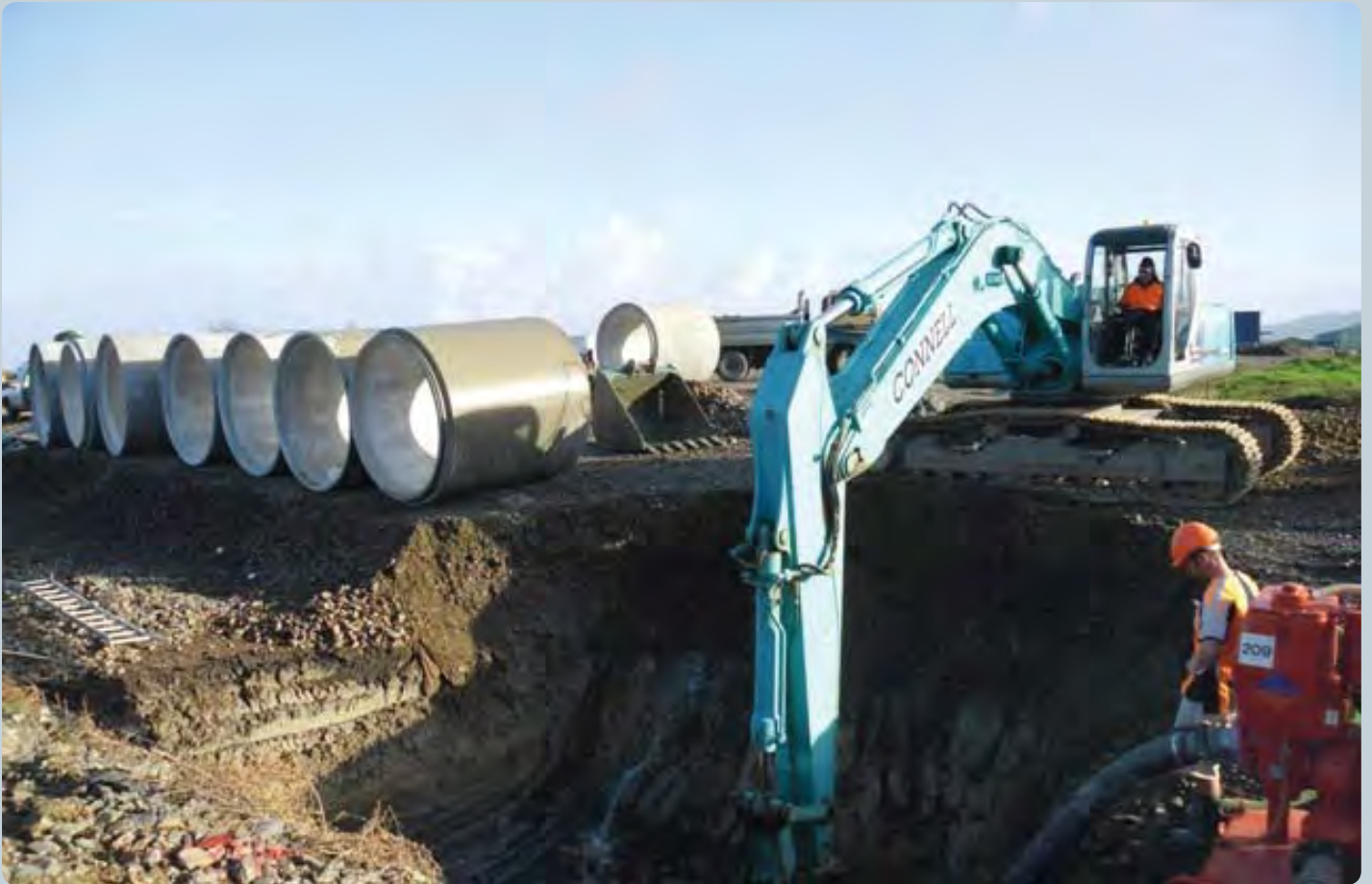
A 2.1 metre culvert is placed under the bridge approach road to provide drainage under the approach road
