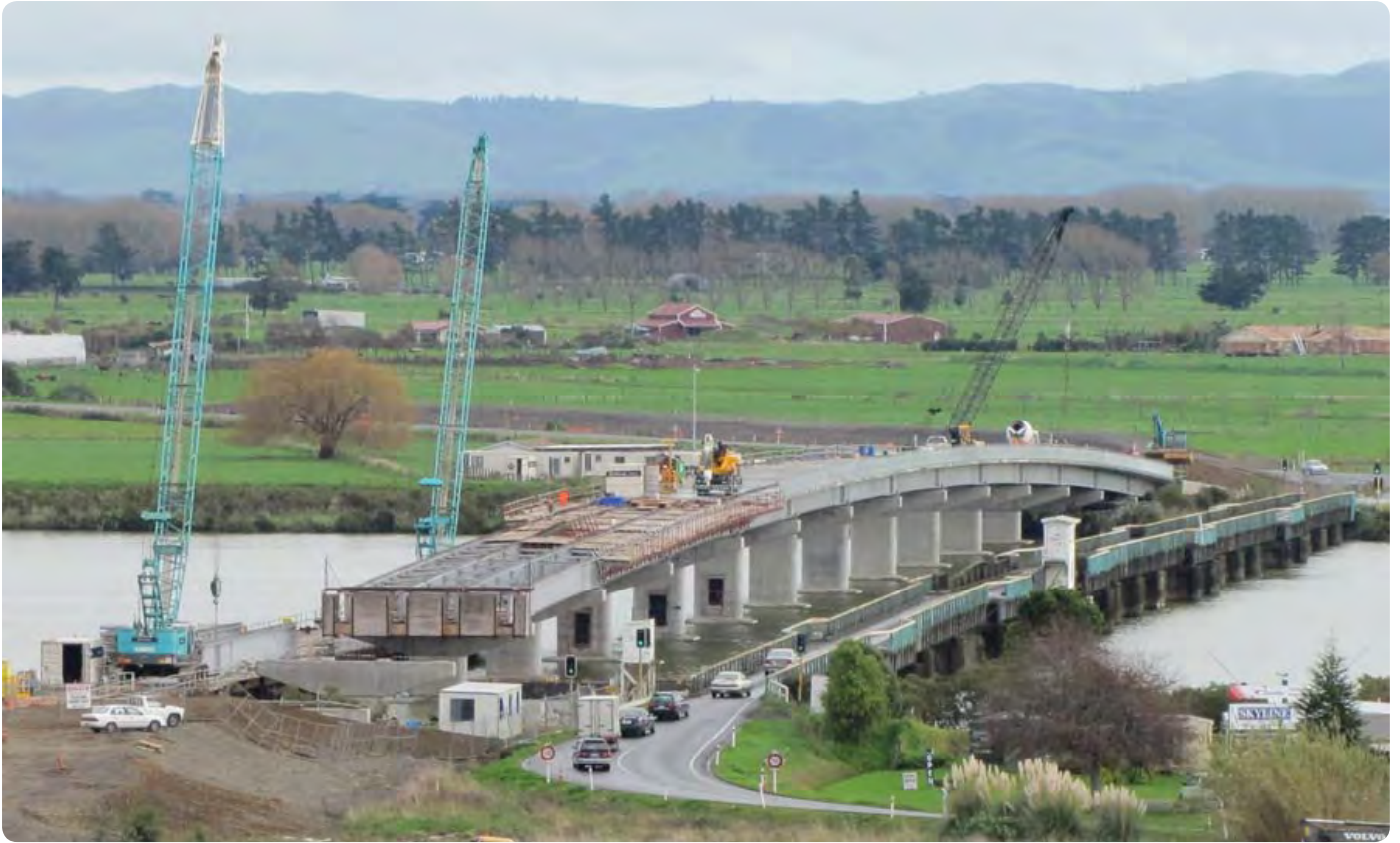
Construction of the bridge is nearing completion. Road construction will follow as soil settlement targets are reached
