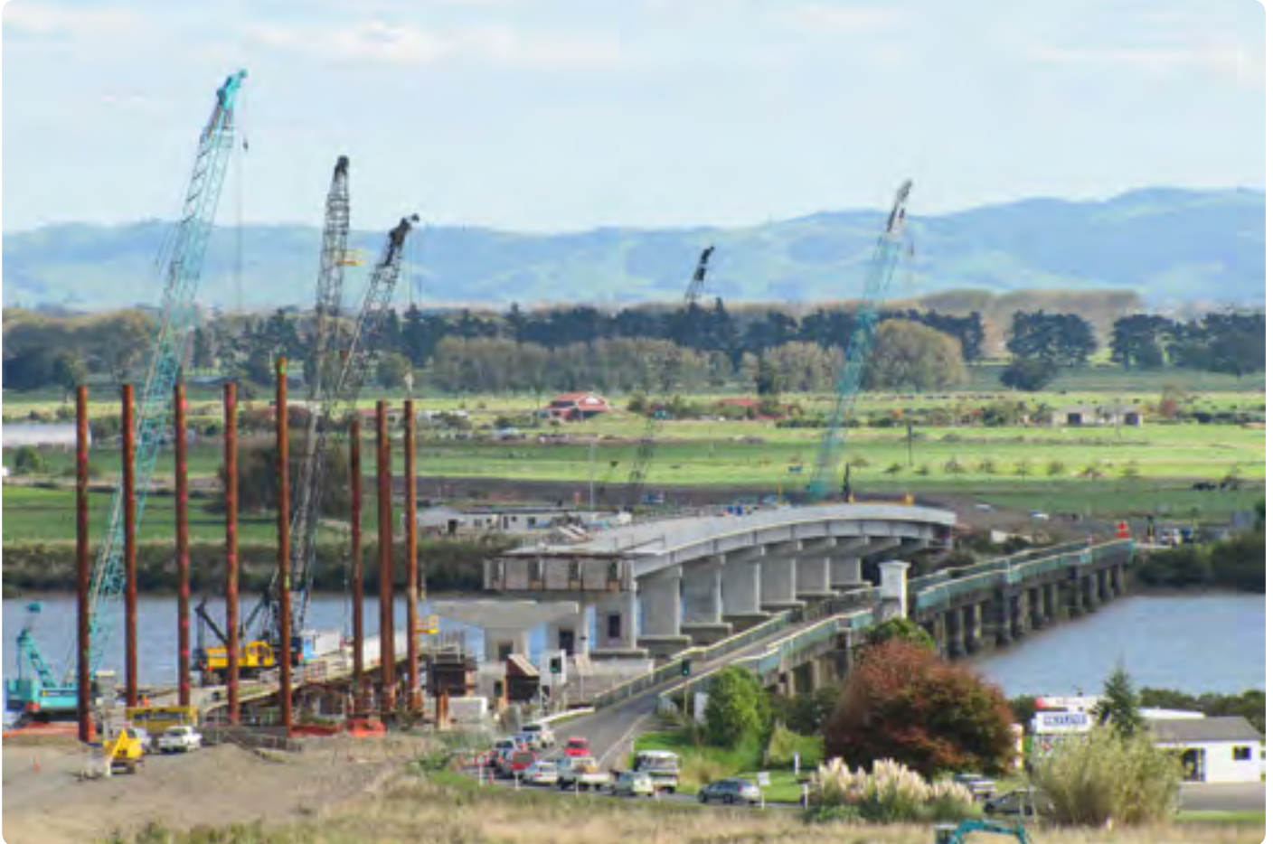
Final piling is completed from the eastern work platform in early May.
