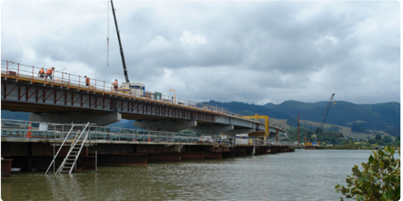
The Kopu Bridge construction site, viewed from the west bank of the Waihou River during flood flows in late January
