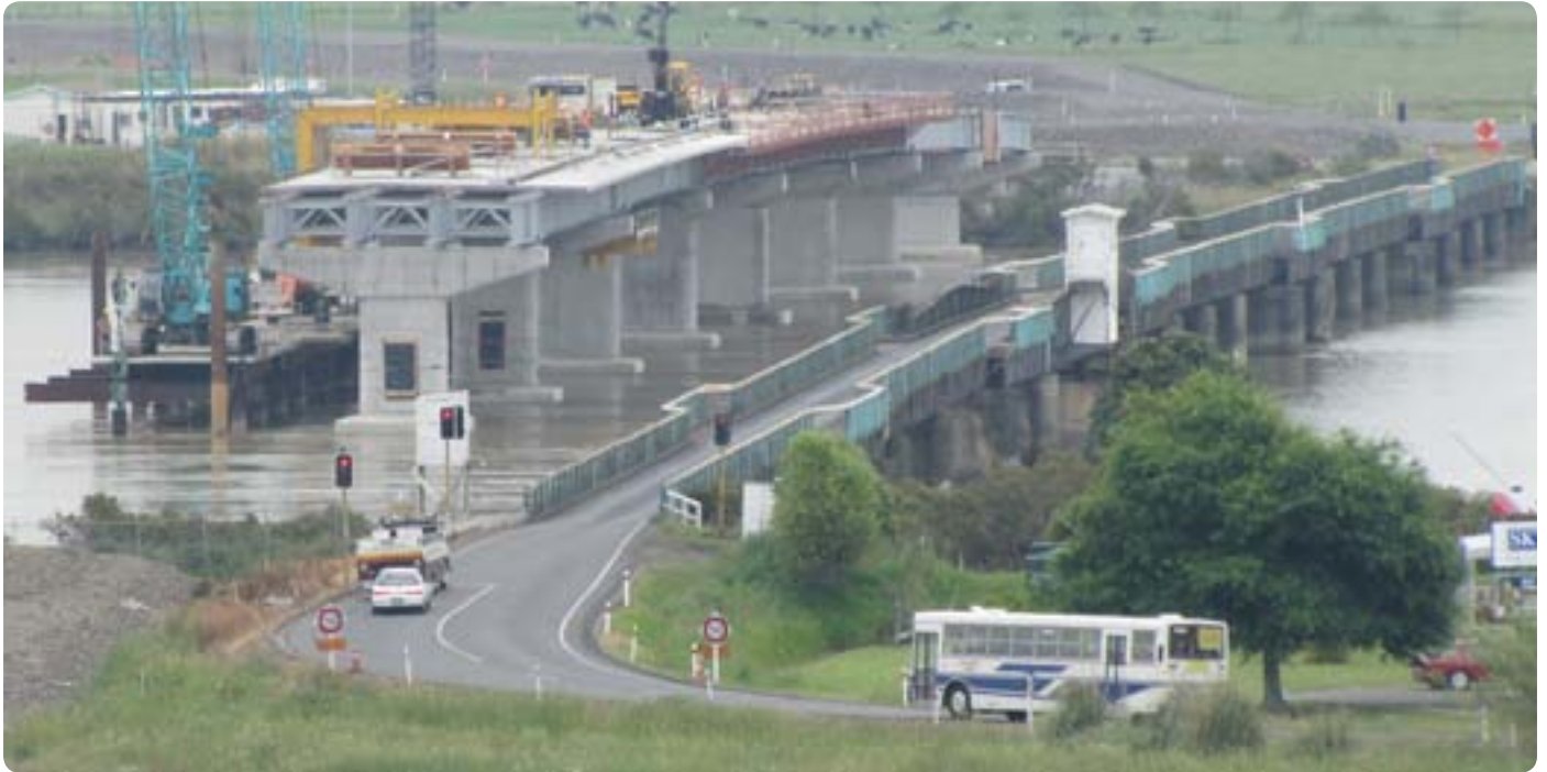
The old and the new – the new Kopu Bridge is taking shape alongside the existing one-lane bridge.
