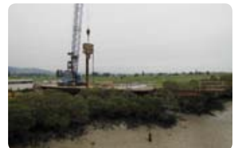
The temporary work platform being built from the eastern bank of the Waihou River.
