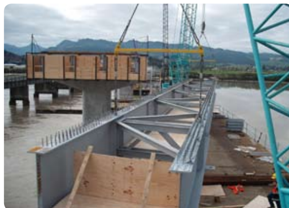
A pair of beams, connected by bracing, are lifted into place on the bridge piers. The wooden floor between the beams provides a temporary working platform for construction staff. Photo supplied by HEB Construction Ltd.
