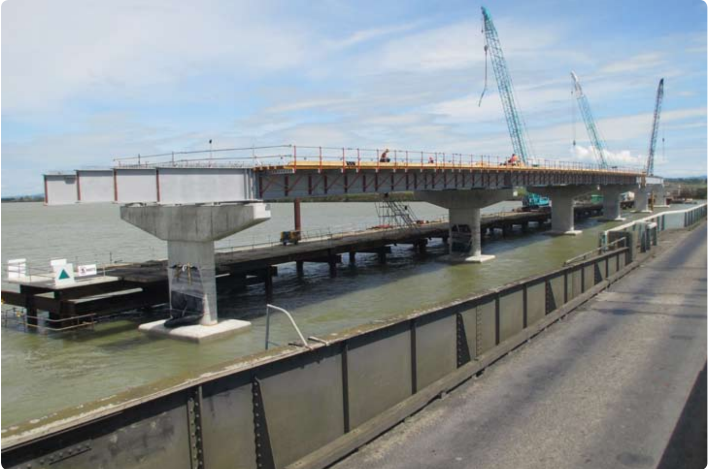
Construction staff are midway through placing the fifth span of bridge beams.
