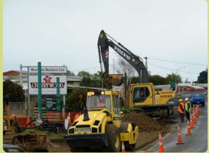
A road construction crew prepares a new lane to connect the existing Ngati Maru Highway (SH26) with the new SH25/26 roundabout.
