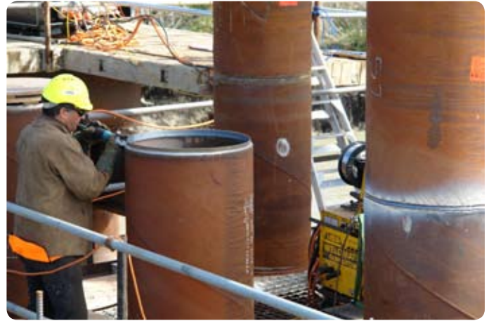
A 36m pile casing has been driven beneath the river. A 24m casing will be welded on top.
