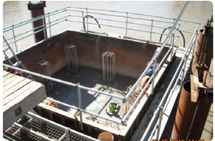
Reinforcing steel protruding from each pile is further reinforced and concrete poured to form a pile cap that will become the foundation for a bridge pier.
