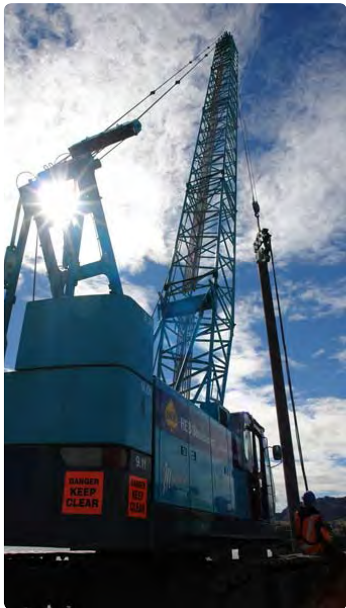
One of the pile cranes being used on the Kopu Bridge project
