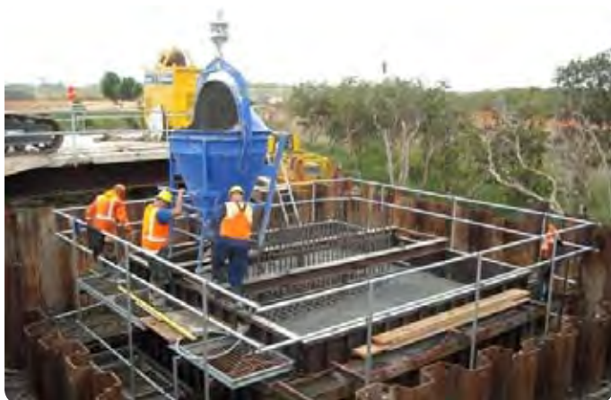
This pilecap will provide the base for a pier to support the new Kopu Bridge
