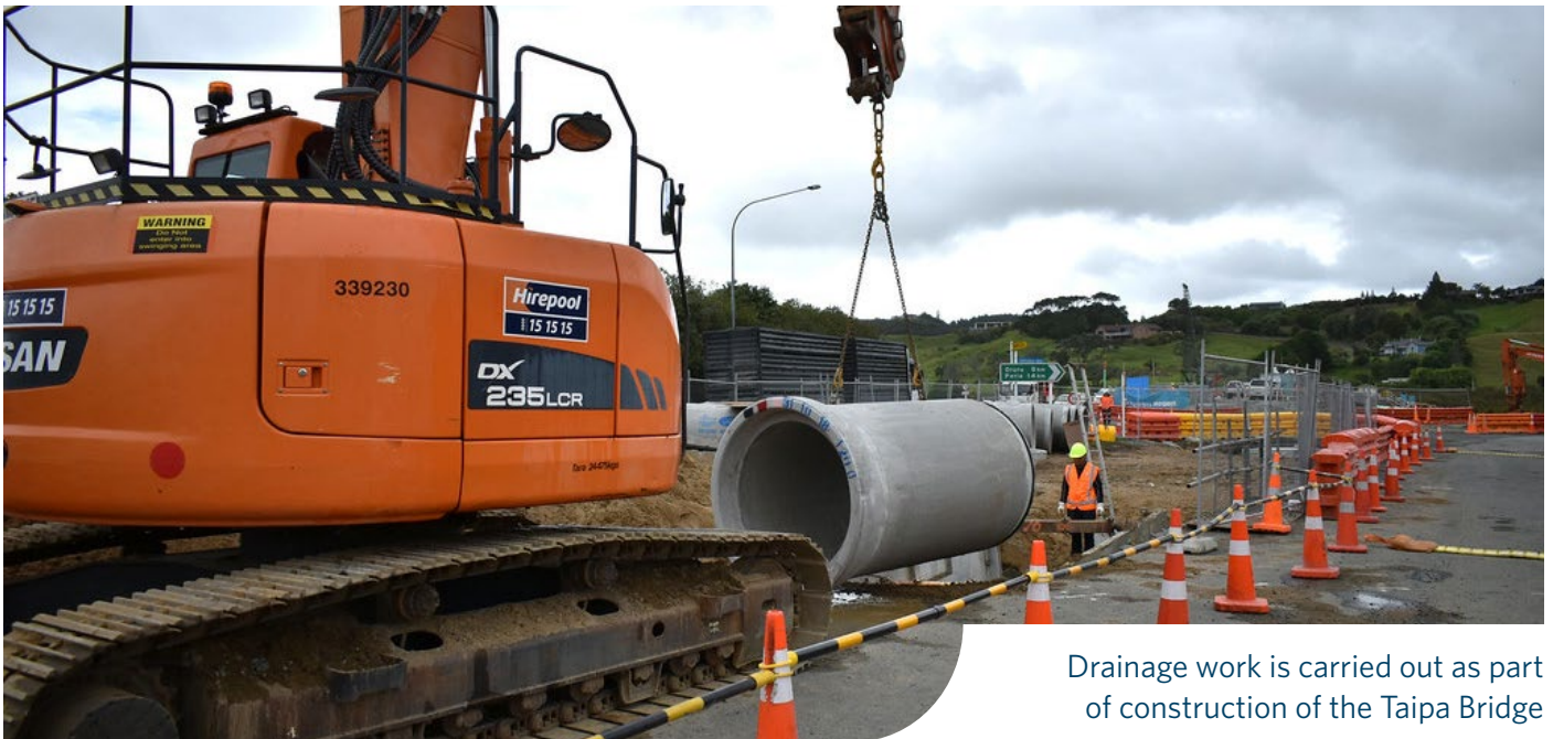
Crews carry out earthworks and prepare the site at the Mangonui end
