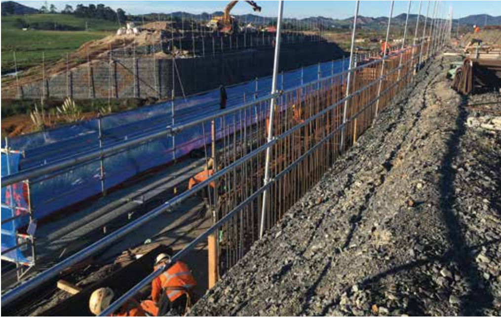
The Northern Interchange bridge abutments will be spanned by beams up to 50 metres long.
