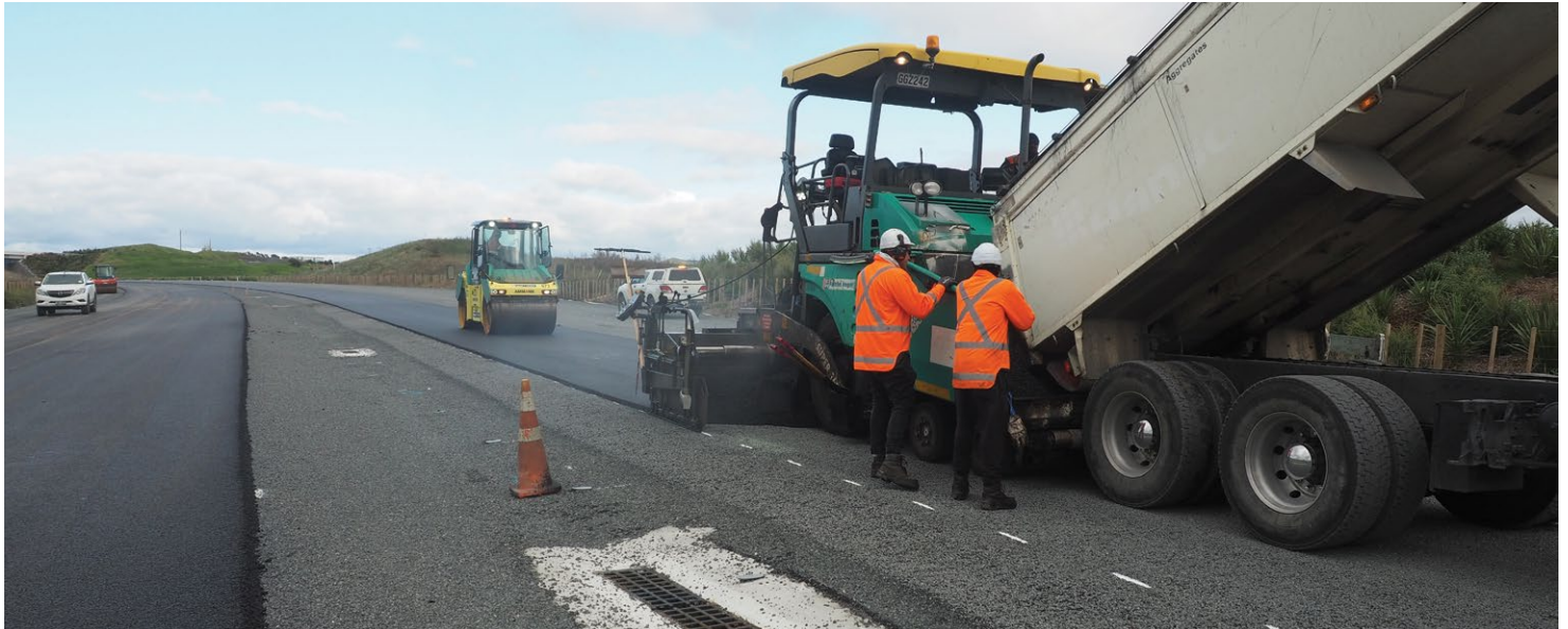
The new highway will open with an asphalt surface which is pictured being rolled out near Ralph Road.
