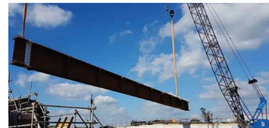
One of the 38 metre central span steel beams being lifted into place.
